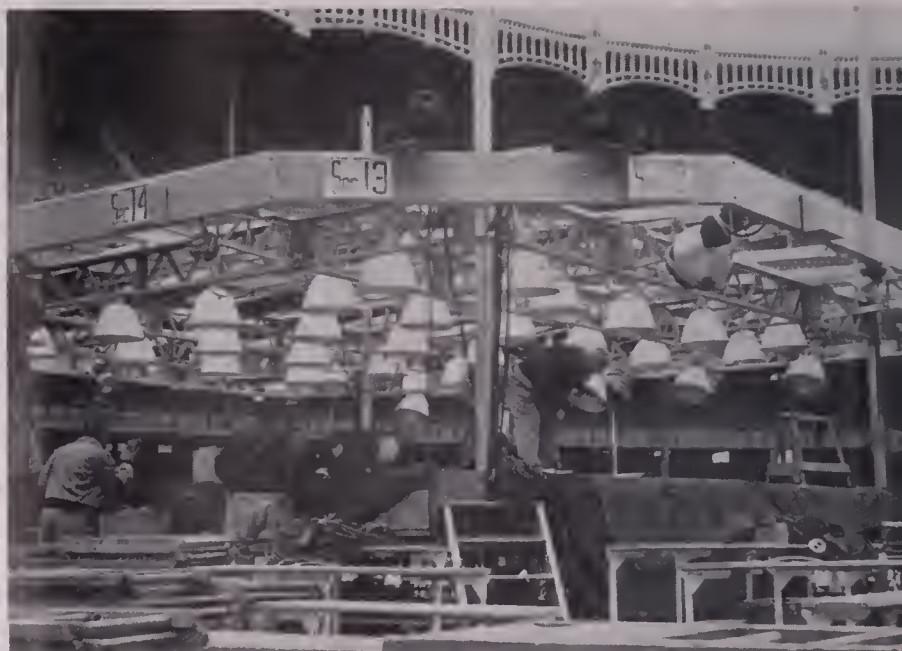
2 TO PROVIDE adequate light for film and TV coverage of bout, thirty-four No. 4 Photofloods mounted in reflectors were installed in framework above the ring. Lamps, which were good for six hours of continuous burning, provided over 600 foot-candles of illumination.
