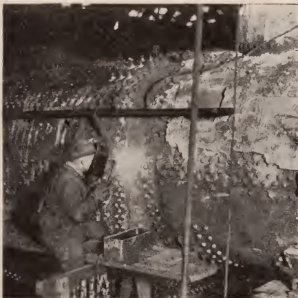
Figure 1—Welding leaky locomotive boiler seam
