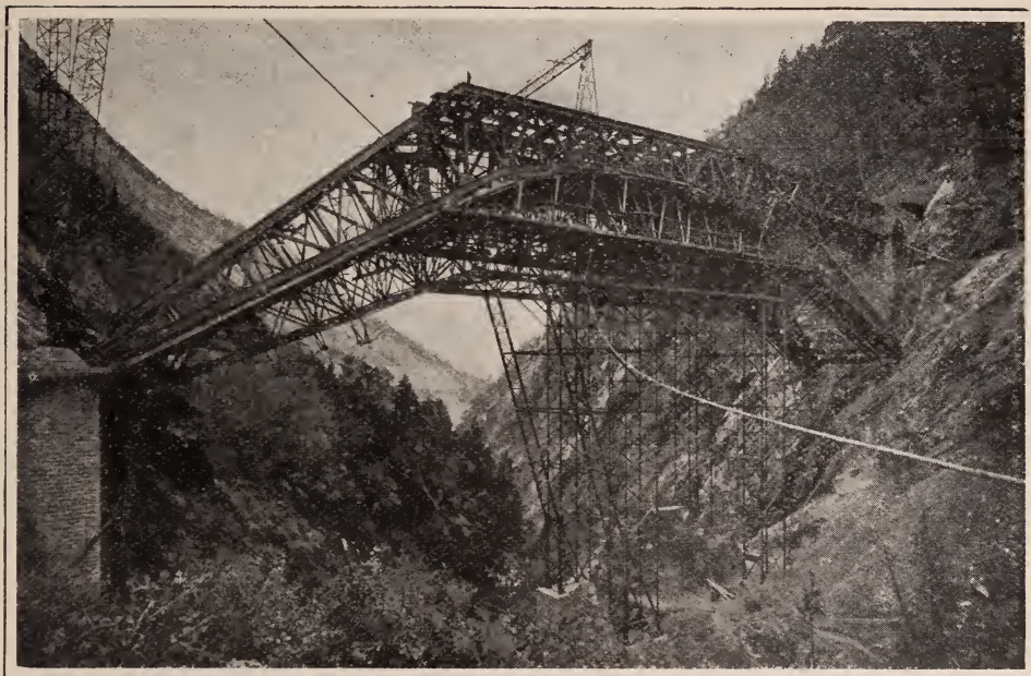
Bietschtai Bridge of unique design, connecting the Bernese Oberland with the Simplon Route
