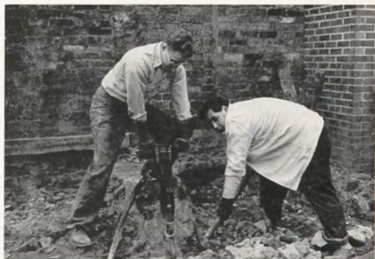
Robert Hoff and Raymond Mazza begin excavation for the new Barracks Rec Hall started last October
