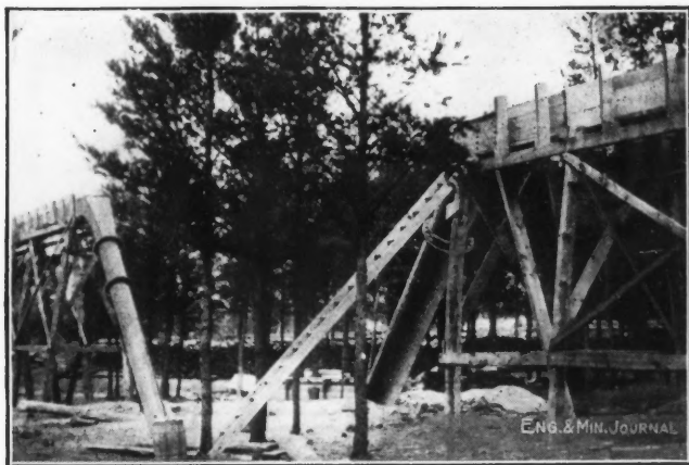
INVERTED SIPHON OF 20-IN. PIPE TO CARRY MINE WATER UNDER RAILROAD TRACKS
