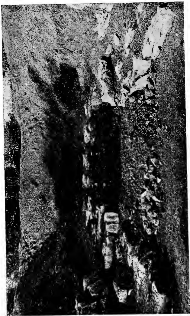
FIG. 4.—A ROCK GARDEN IN THE MAKING. THE DRAINAGE FOR THE CENTRAL MOUND IS WELL SHOWN.
