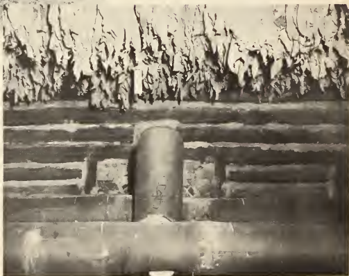
Figure 23.--Inside view of a curing barn showing metal flues that carry heat from a furnace. →
