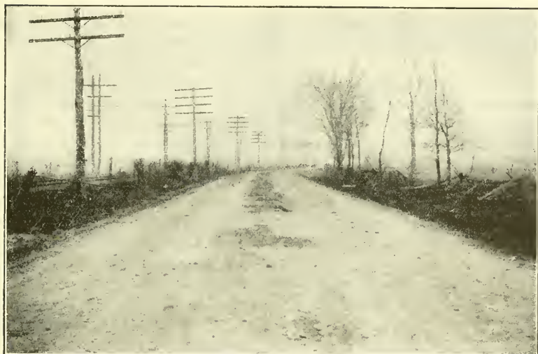
FIG. 1.—WATERFORD ROAD, WATER-BOUND MACADAM THROWN BY FROST, MARCH 30TH, 1910.
