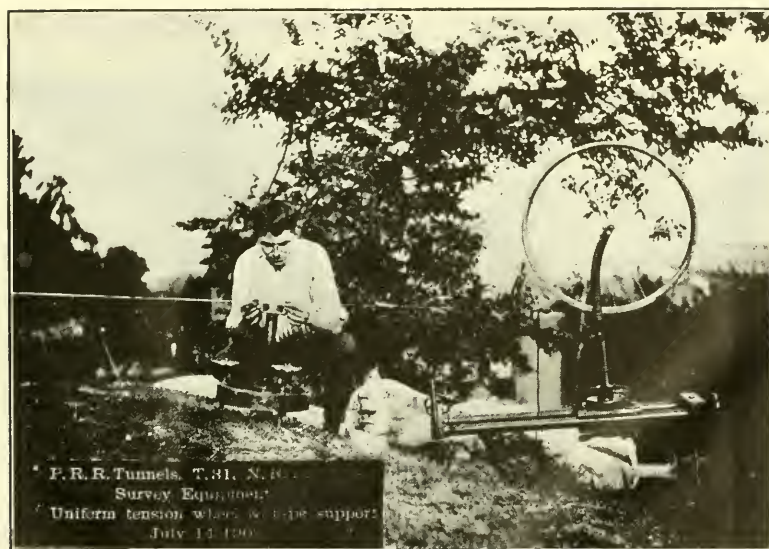
FIG. 11.—UNIFORM TENSION WHEEL AND MOVABLE STATION POINT, OR "SPIDER," USED IN BASE LINE MEASUREMENTS. PENNSYLVANIA RAILROAD TUNNELS.
