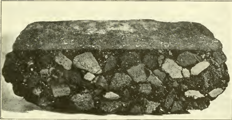
FIG. 8.—BITUMINOUS MACADAM ROAD, PENETRATION METHOD, STANDARD MACADAM ASPHALT BINDER, NEW YORK STATE SPECIFICATIONS. HUNTINGTON-FARMINGDALE ROAD, LONG ISLAND, BUILT 1909. SAMPLE TAKEN FROM ROAD, NOVEMBER, 1911.
