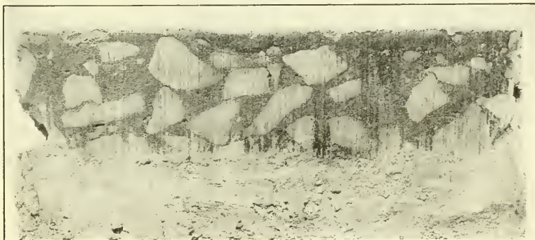
FIG. 12.—SEC. 3.—BITUMINOUS PAVEMENT BUILT BY MACHINE-MIXING METHOD. 2 PARTS TRAP ROCK PASSING 1¼-IN. RING, WITH MAXIMUM OF 5% DUST, 1 PART SAND, AND 8% BERMUDEZ ASPHALT.
