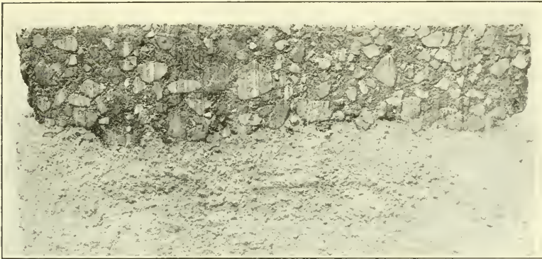
FIG. 10.—SEC. 1.—BITUMINOUS PAVEMENT, BUILT BY MACHINE-MIXING METHOD. 73% PAVING GRAVEL, 19½% SAND, 1½% DUST, AND 5.4% BERMUDEZ ASPHALT.
