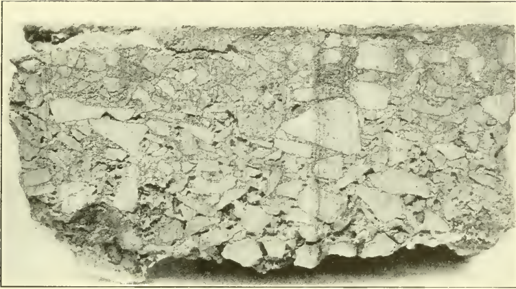
FIG. 20.—SEC. 9C.—BITUMINOUS PAVEMENT, BUILT BY HAND-MIXING METHOD. THREE PARTS \frac{3}{4} -IN. TRAP ROCK, 1 PART CHIPS, AND 7% MIXTURE OF TAR AND 10% BERMUDEZ ASPHALT.
