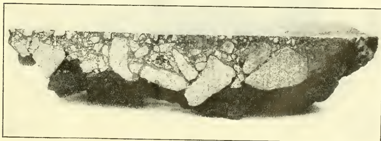
FIG. 26.—SEC. 15.—BITUMINOUS PAVEMENT, BUILT BY PENETRATION METHOD. 1\frac{1}{2} -IN. TRAP ROCK, ROLLED TO A DEPTH OF 2\frac{1}{2} IN., 2.3 GAL. TARVIA APPLIED. LAYER OF CHIPS ROLLED. \frac{3}{4} GAL. TARVIA APPLIED. FINISHED BY ROLLING LAYER OF CHIPS.
