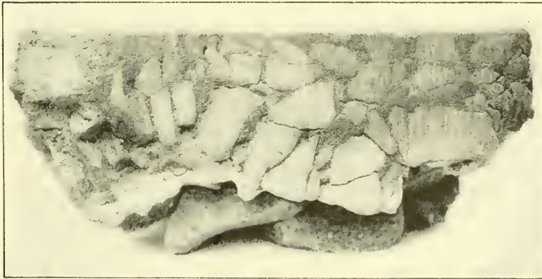
FIG. 28.—SEC. 17.—BITUMINOUS PAVEMENT, BUILT BY PENETRATION METHOD. 1½-IN. TRAP ROCK ROLLED TO A DEPTH OF 6 IN., 1½ GAL. STANDARD OIL COMPANY'S BINDER B APPLIED, LAYER OF ¾-IN. TRAP ROCK ROLLED, 1.1 GAL. BINDER B APPLIED. AFTER WHICH LAYER OF CHIPS WAS ROLLED.
