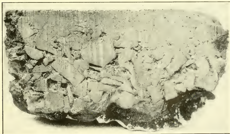
FIG. 17.—SEC. 8.—BITUMINOUS PAVEMENT, BUILT BY HAND-MIXING METHOD. THREE PARTS \frac{3}{4} -IN. TRAP ROCK, 1 PART CHIPS, AND 6\frac{1}{2}\% TARVIA X.
