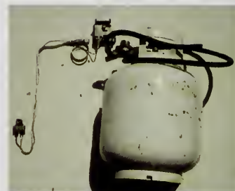
a Pilot light propane heater
