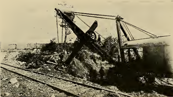
STARTING AN OPEN PIT MINE. THE EARTH COVER- ING IS BEING REMOVED
