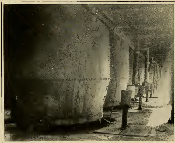
LOWER HALF OF A "BATTERY" OF MODERN GAS PRODUCERS
