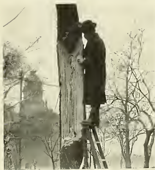
Too long neglected; wind storm split it
