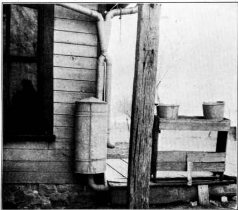
FIG. 5.—Galvanized-iron charcoal filter and rain-water switch. Water passes into a dug well. Not a desirable installation.
