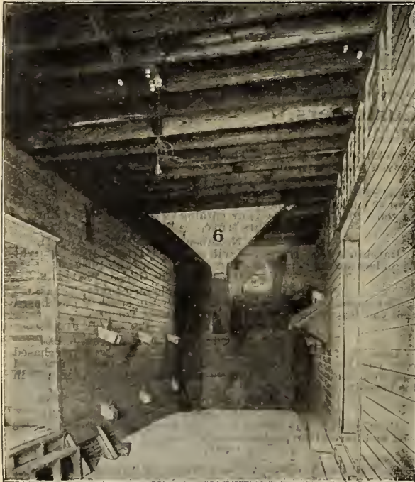
A SECTIONAL VIEW OF DRIVEWAY through our seed house; also showing outlet of our large storage bins.
