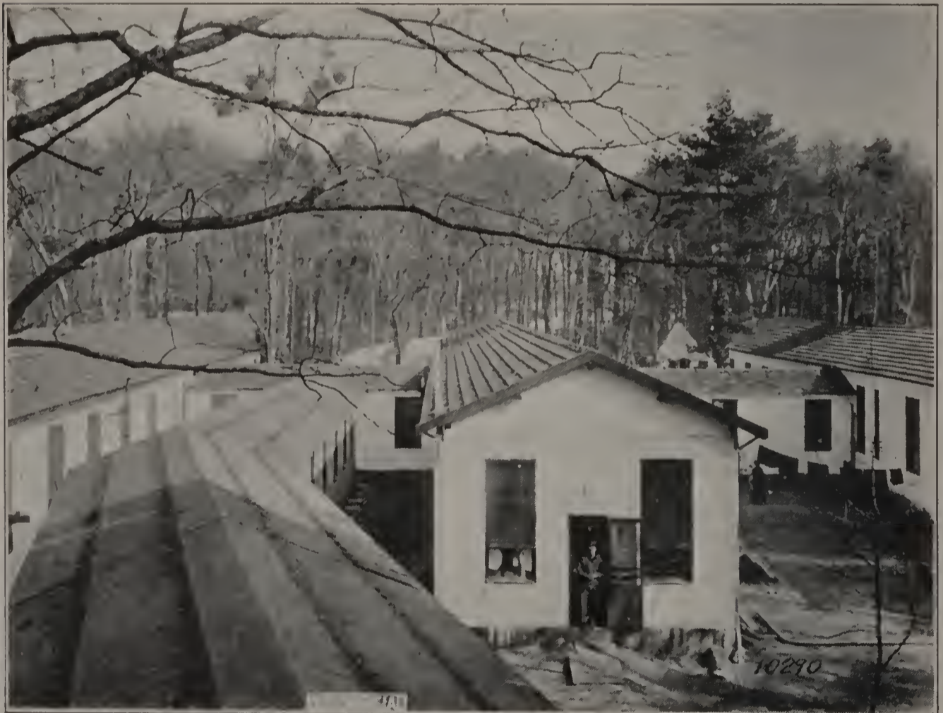
FRENCH BARRACKS SHOWING IN THE BACKGROUND CORRIDOR OF THE NEW CONSTRUCTION ON THE COLIN ESTATE
