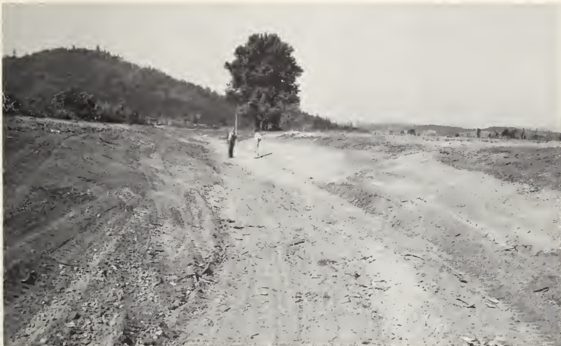
Figure 43.--A channel realignment job is nearly completed on Evergreen Creek, subbasin 6, Middle Willamette River Basin, Oreg., 1961. SCS photo.7-1164-1
