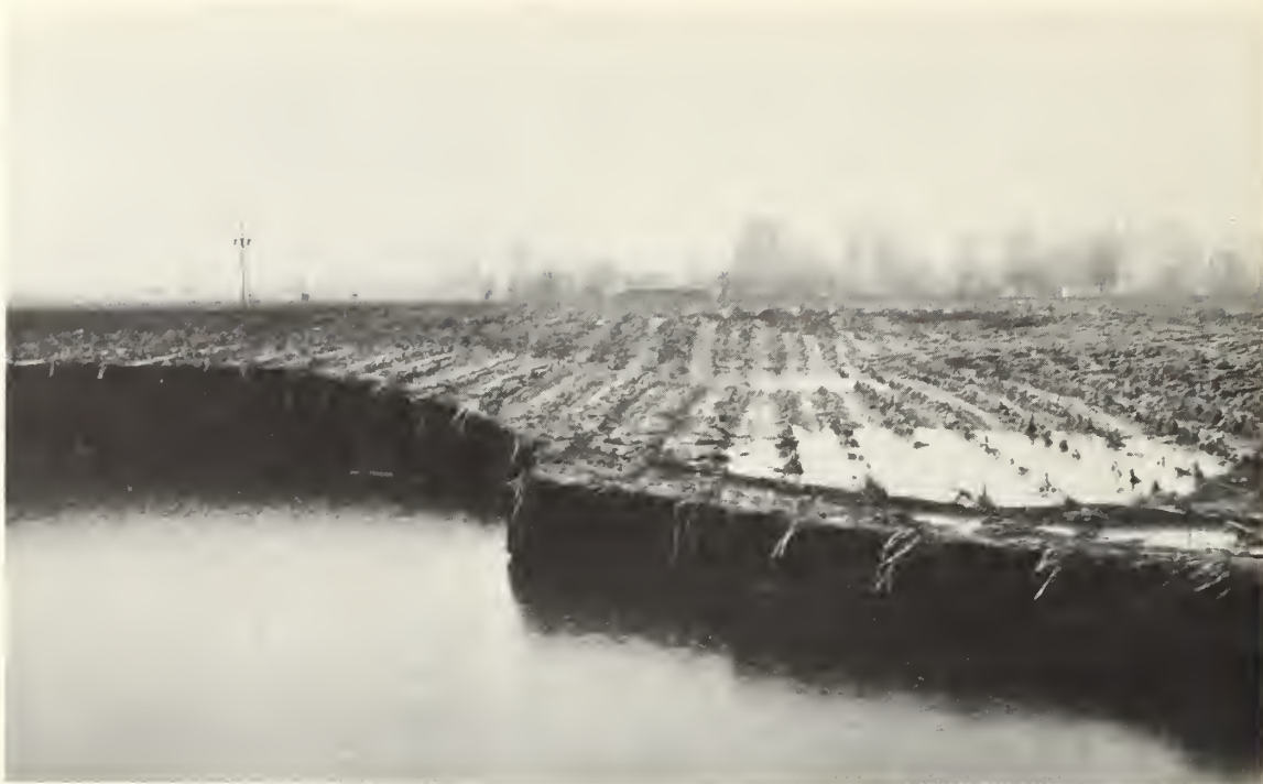
Figure 31.--This bank erosion is on Thomas Creek, sub-basin 5. The water is about 10 feet deep and the bank about 6 feet above the water line. SCS photo. scs 7-602-6
