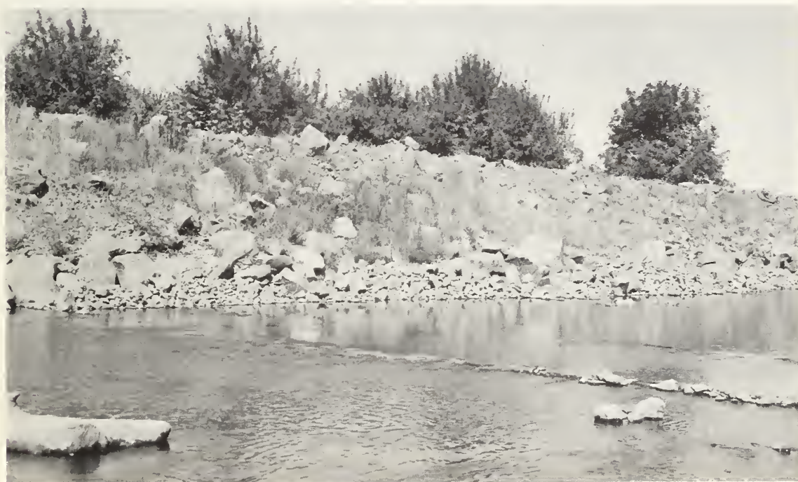
Figure 44.--This rock riprap on Thomas Creek was placed in 1954 and 1955, subbasin 5, Middle Willamette River Basin, Oreg. SCS photo.7-605-1
