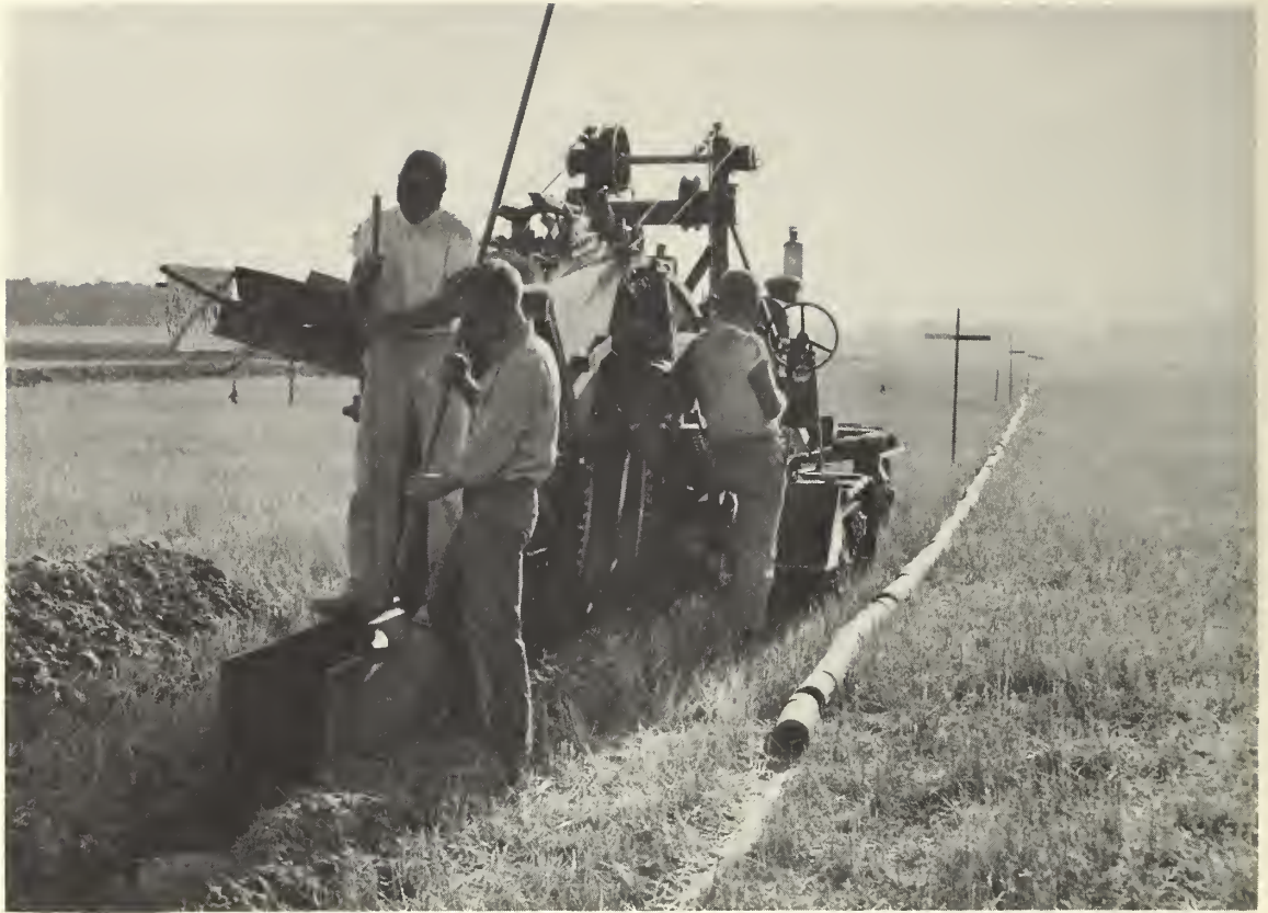
Figure 42.--Clay tile is laid in trenches spaced in a pattern for good drainage, subbasin 6, Middle Willamette River Basin, Oreg. SCS photo. 7-883-11
