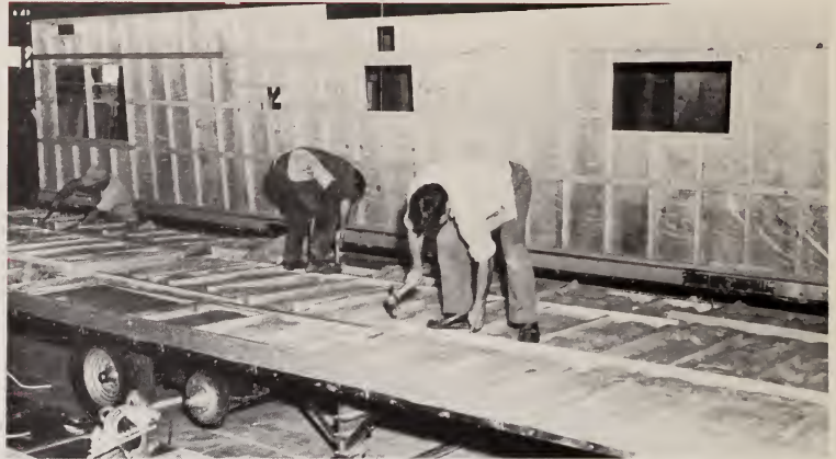
"Polythene" vapor barrier and special insulation reinforce Esta-Villa coaches against Western Canada winter weather.
