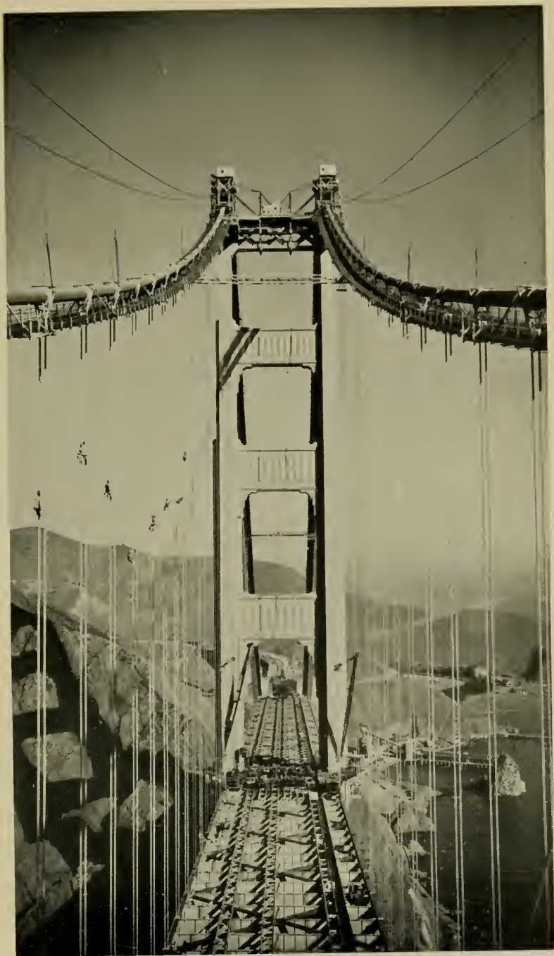
SUSPENDED FROM THE CABLES IS THE STEEL FLOOR STRUCTURE UPON WHICH THE CONCRETE ROADWAY WAS LAID.
