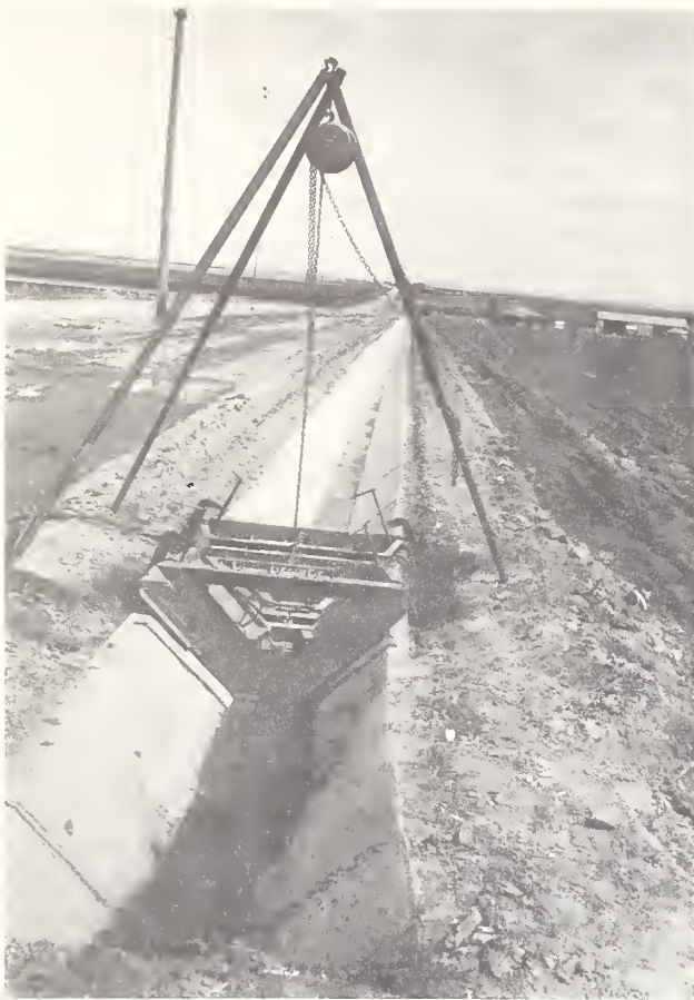
Figure 5. Form in place for casting a flume with a raised bottom. Note end extension section, tripod and chain hoist for handling the form, and "C" clamps which secure the form to existing lining.
