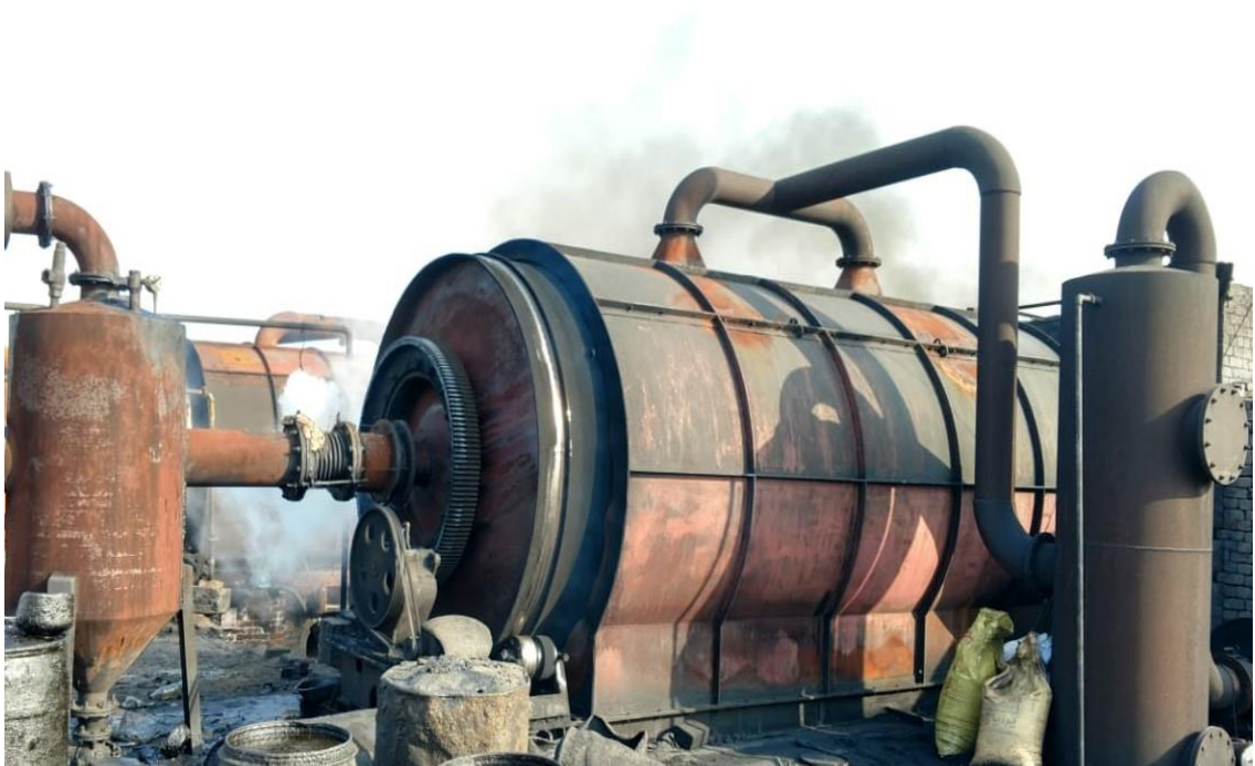
Fig. 7.2: Waste Tire Pyrolysis Plant
