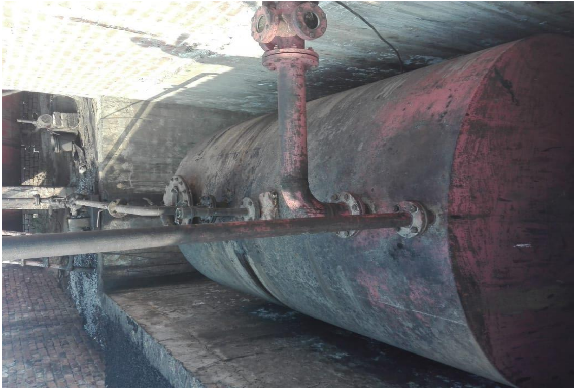
Fig. 7.3: Oil Collector Tank
