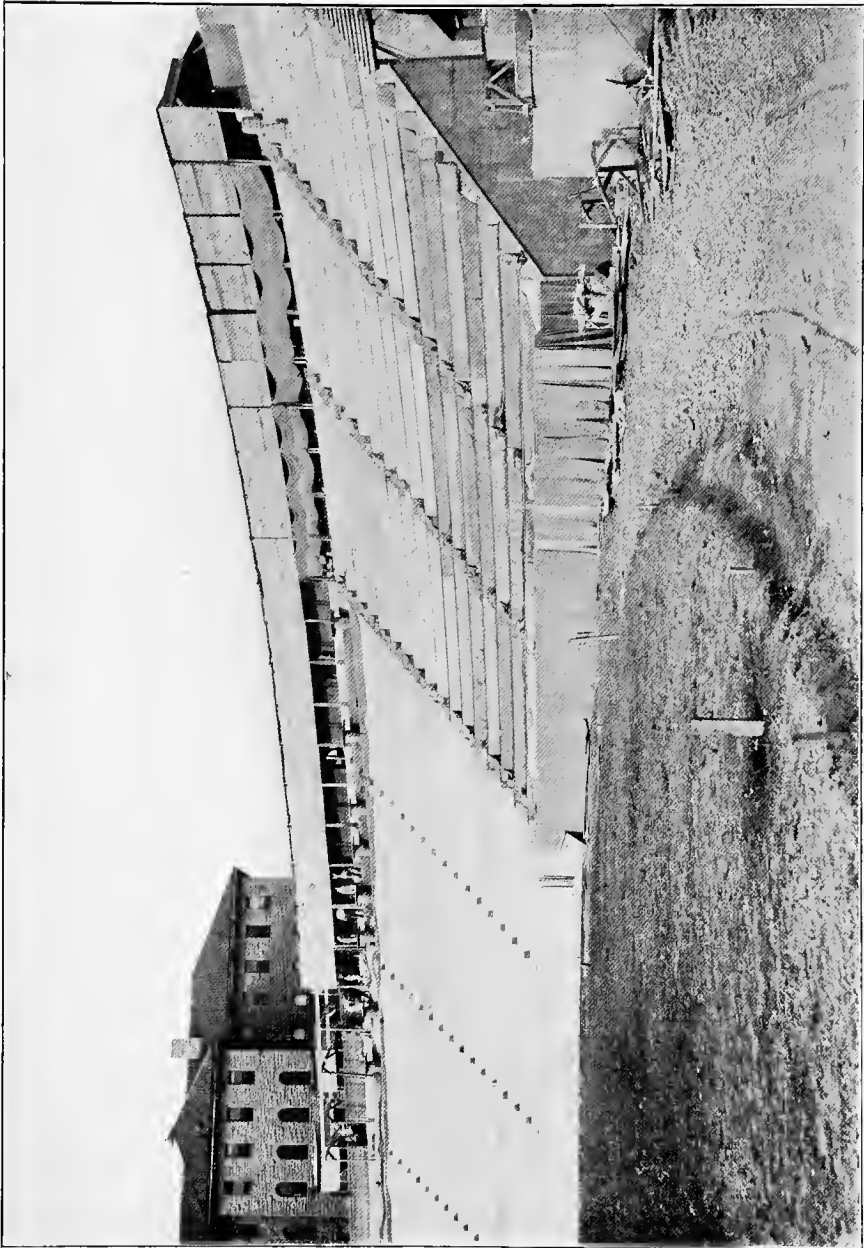
This picture shows the cement finishers working under the sheds on the small wall at the top of the seats. It also shows the manner of covering the seats with burlap and sand, after they are finished, to prevent the cement from setting too rapidly.
