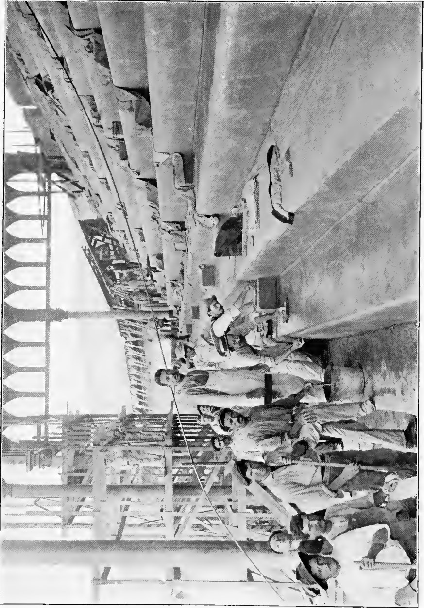
This view shows the method of applying the cement finish to the rough concrete seats.
