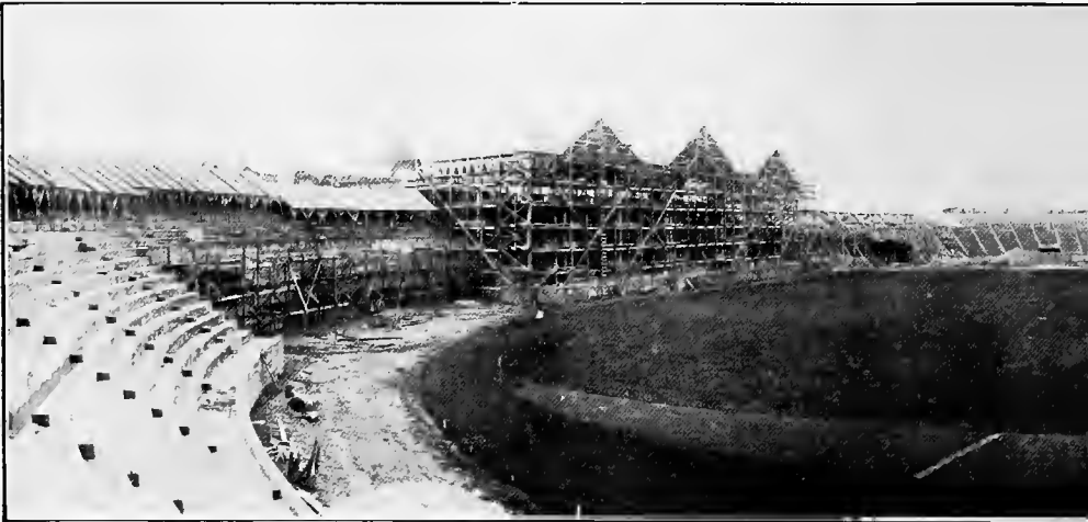
View looking West. Note the main arch of the entrance in the center of the stadium. The clear span of this arch is 40 feet, obtained by noting that this arch in the distance is 40 feet clear span.
