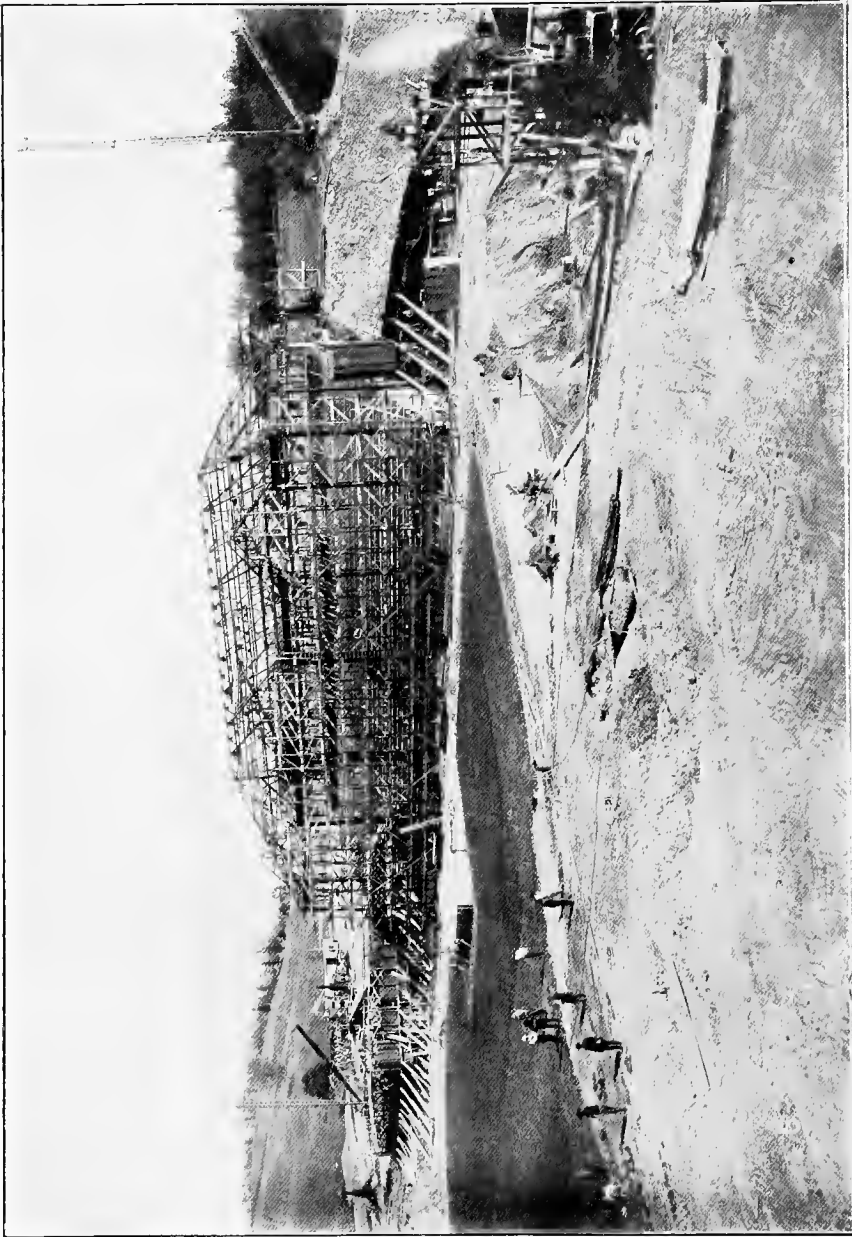
This picture shows the Grand Stand scaffolded ready for cement work, and in the upper left hand corner, it shows the steel derrick set up for hoisting excavated materials in cars onto the trestle, from which point they run by gravity into the valley.
