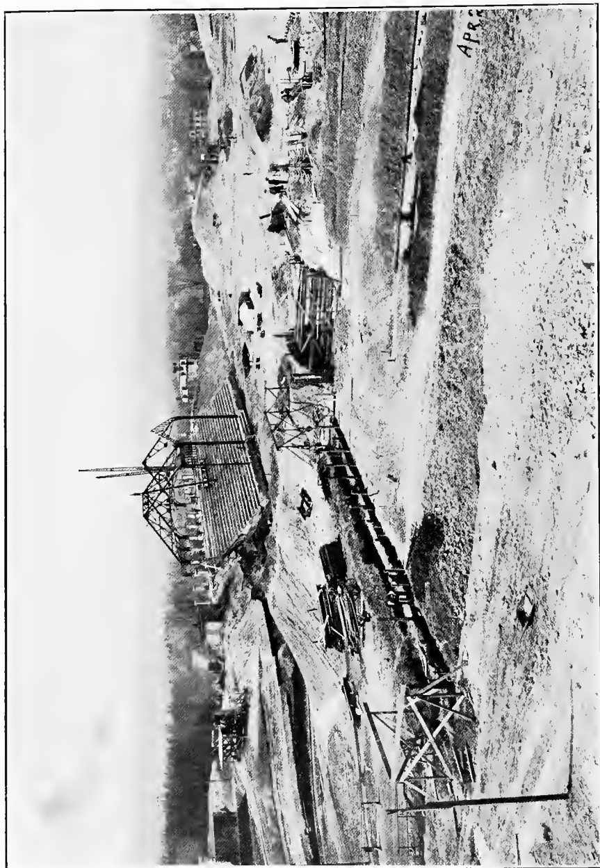
This picture shows the steel derrick erecting the structural steel over the Grand Stand, also the excavation for the rear wall of the Gymnasium and for the tunnel which is to connect the basement of the Gymnasium with the field of the Stadium.
