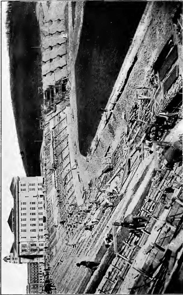
To the left can be seen the manner of forming the seats and the supporting girders. In the upper left hand corner, in the distance, is Sims Hall, Men's Dormitory Building, which was erected last year by the Consolidated Engineering & Construction Company.
