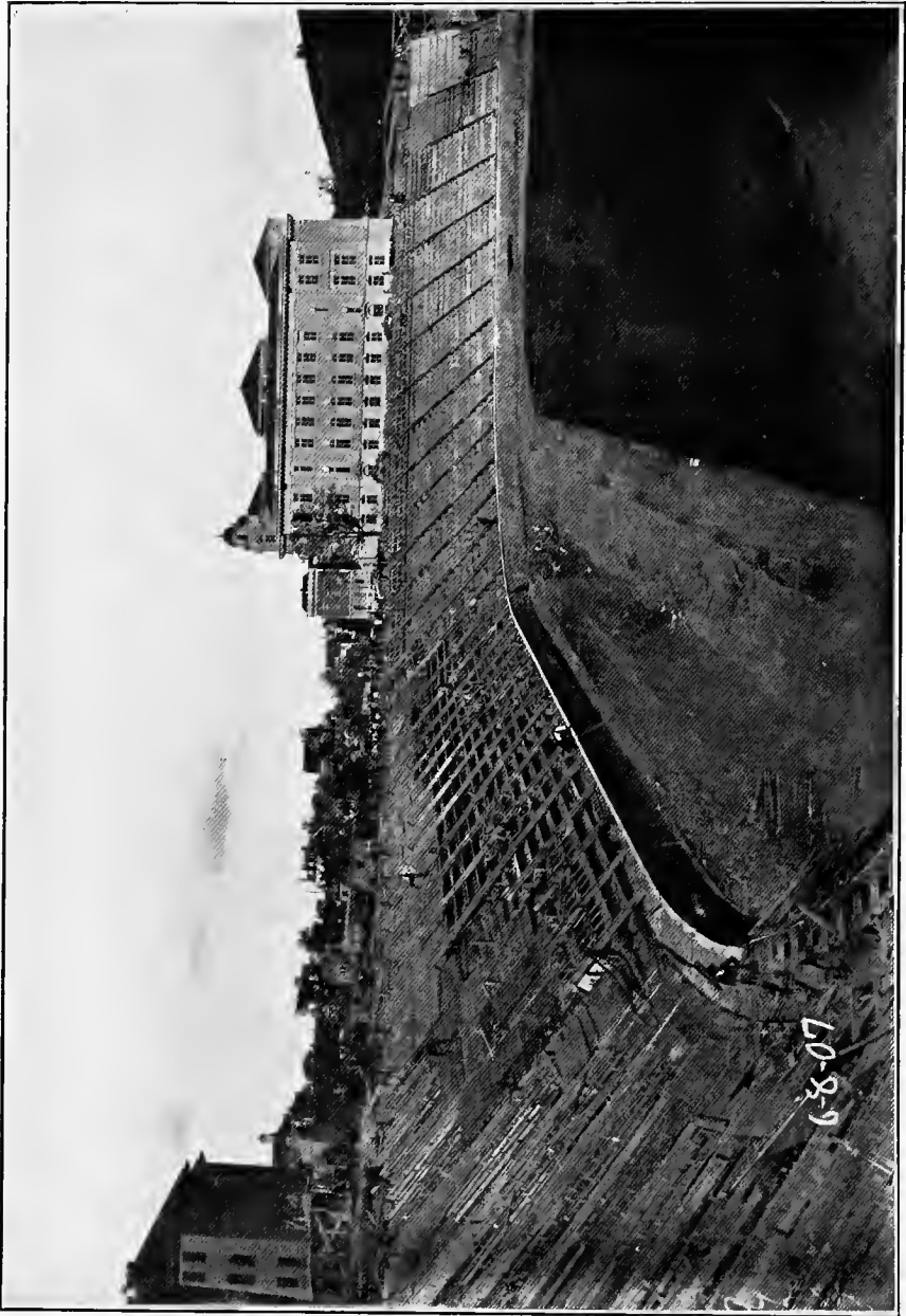
This picture shows the seats under construction over the tunnel and on the North side.
