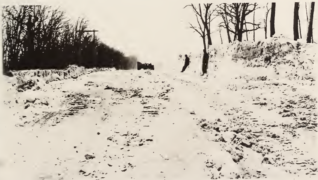
FIGURE 12. A ROADWAY CLEARED TO A GENEROUS WIDTH WITH THE HEAVIER TYPE OF ROTARY PLOW.
