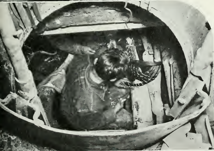
This splicer in Providence, R. I., is drying out cables while the manhole is still partly flooded.
