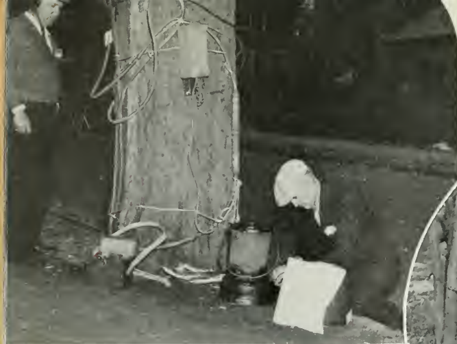
Using a tree as a telephone pole to provide emergency service for the Melrose, Mass., Hospital.
