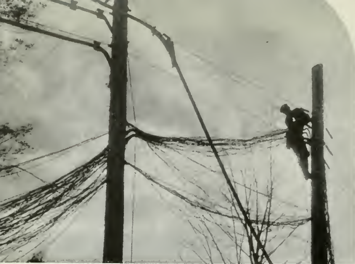
Untold miles of twisted pair were quickly run to restore temporary links in important circuits. This scene is in Eastern Connecticut.
