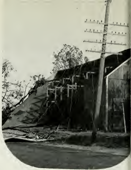
Most of this barn blew through the telephone line at Wapping, Conn.
