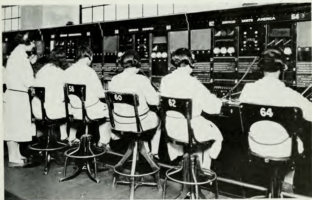
CALLS TO AND FROM NORTH AMERICA ARE HANDLED AT THIS SECTION OF THE LONG DISTANCE SWITCHBOARD IN BUENOS AIRES.
