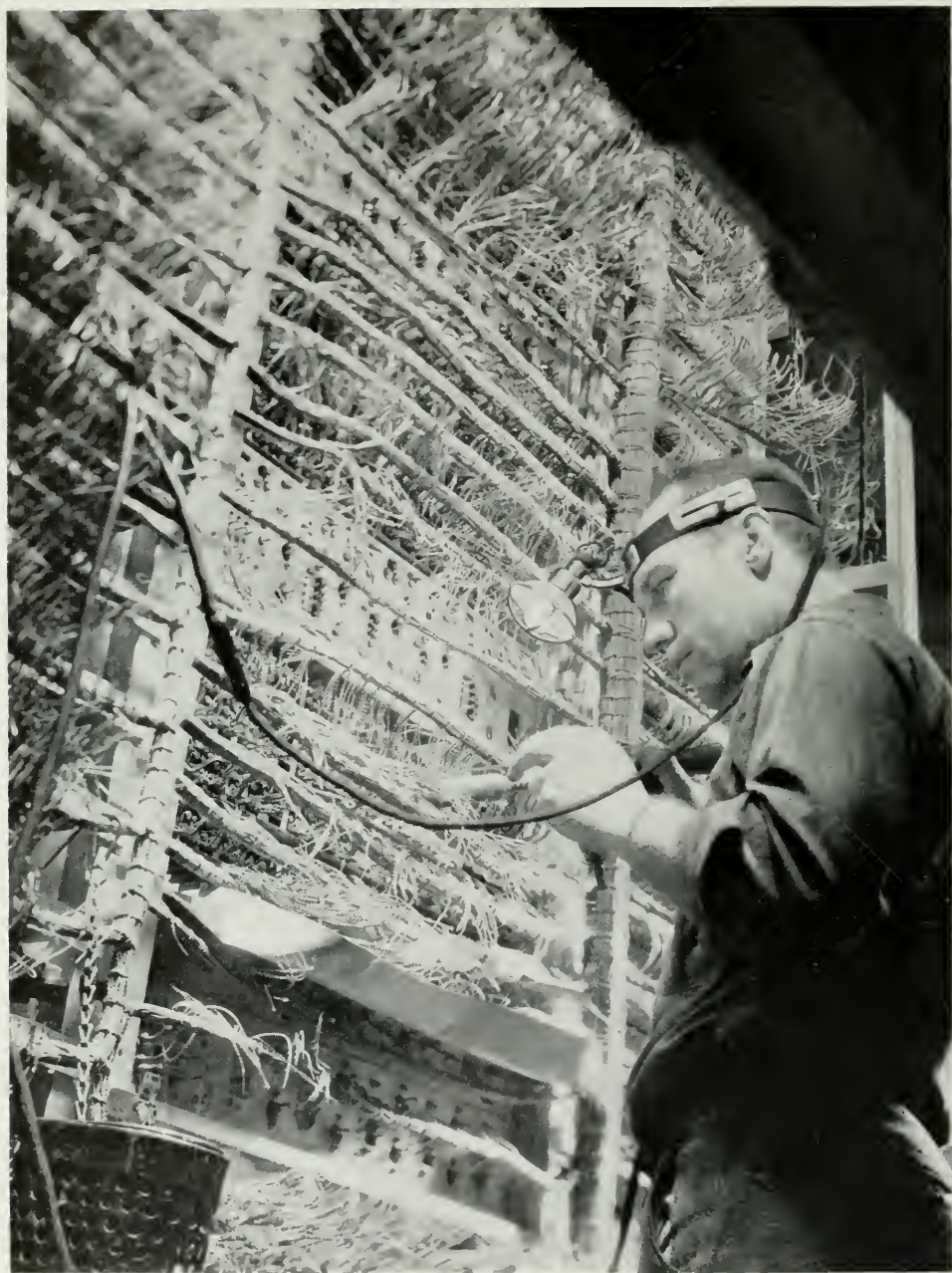
Under the sure touch of the craftsman, this bewildering maze of wire will shortly be converted into a neat and orderly bay of relay rack in a central office, with every last wire soldered to its correct terminal.
