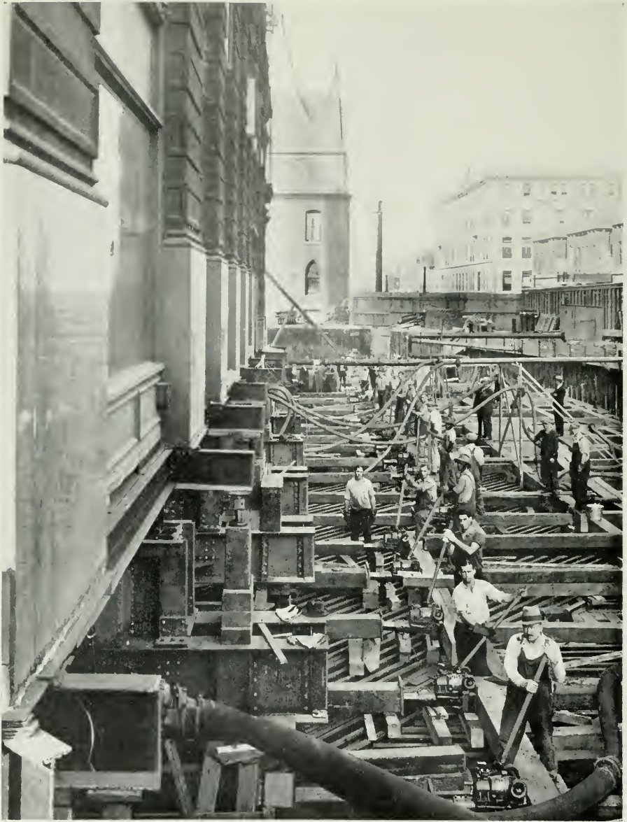
FIG. 5. EIGHTEEN MEN WITH JACKS PUSH 8-STORY, 11,000 TON BUILDING. THIS PICTURE SHOWS THE START OF THE STRAIGHT MOVE SOUTH.
