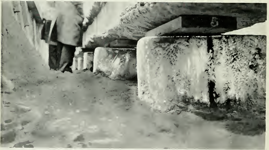
FIG. 8. USING BLOCKS OF ICE TO GENTLY LOWER OCCUPIED TELEPHONE CONDUIT IN ORDER TO PERMIT CHANGES IN HIGHWAY GRADE NEAR FLOYD BENNETT AIRPORT, NEW YORK.
