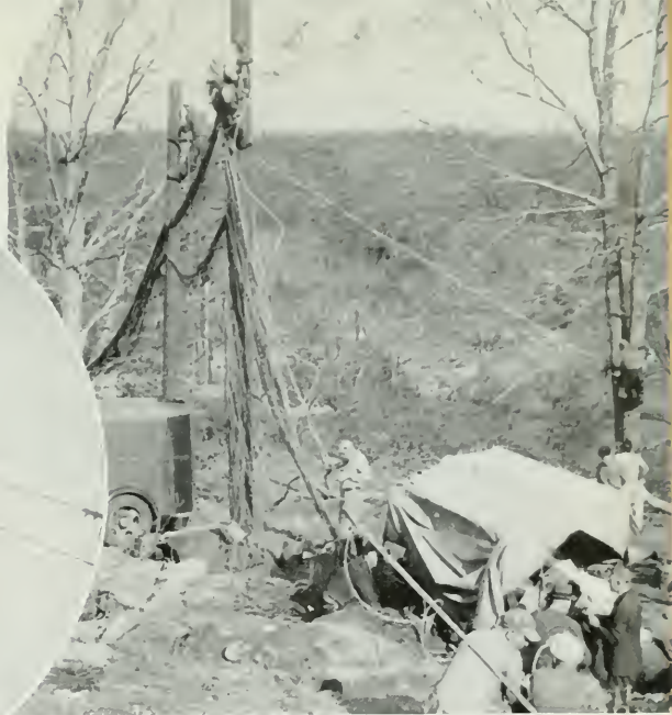
Right: Long Lines men splicing temporary twisted pair at an important cable break at Atwoodville, Conn.
