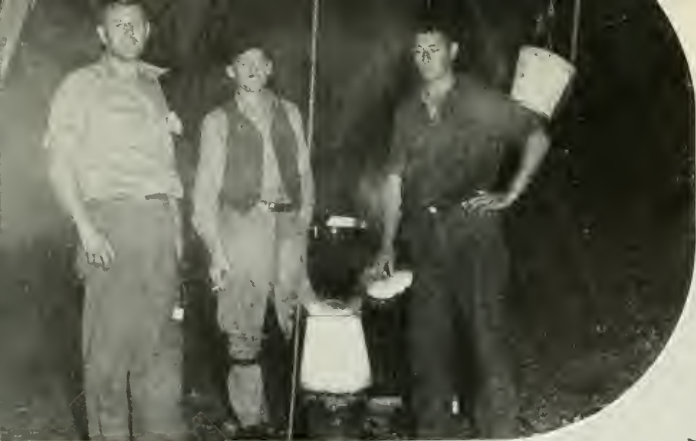
Left: Work goes on far into the night. These Southern New England men are making temporary repairs on a New Haven-New London toll cable at Lyme, Conn.
