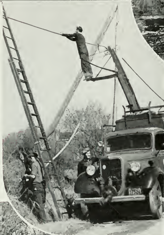
A Pennsylvania Bell crew doing restoration work at Narragansett pier, R. I.
