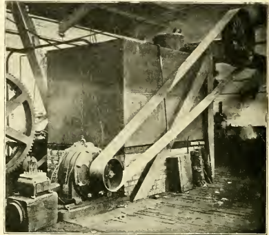
TYPE "C" MOTOR OPERATING AIR COMPRESSOR.
