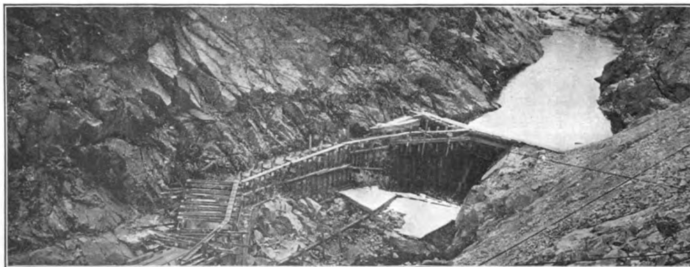
At last bed-rock was dry. The river was conquered. Twenty feet above its bed it hugged the wall of the gorge in a flume, squeezed to one side to make room for the gigantic dam that was to rise three hundred feet above the granite base
