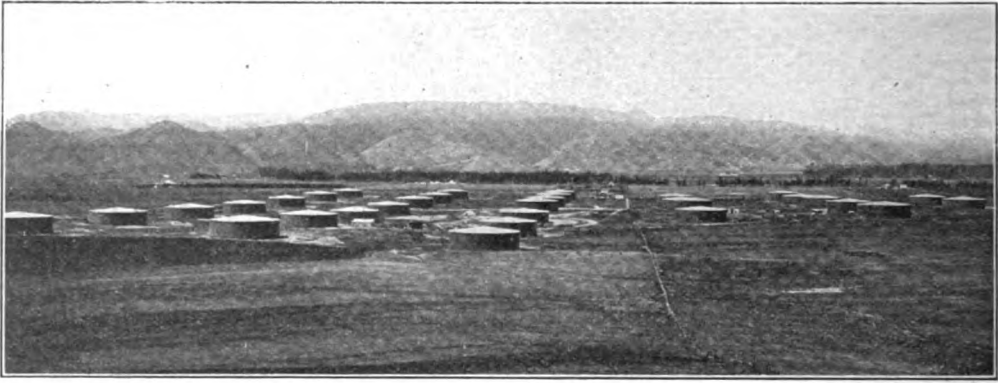
A "tank farm." The increasing output of high-gravity petroleum in the immense California oil fields, the growing number of plants that squeeze every drop of gasoline out of the heavy oil and out of natural gas before these materials are burned under the boilers, have helped to reduce the cost of automobile fuel in the West
