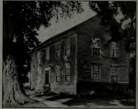
In contrast, the Pink House across the way, so-called because of the remains of a prehistoric coat of pink paint, shows cornices in decay and numerous patches.
