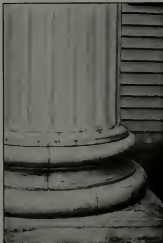
When paint loses its protective grip on a column base, moisture enters, and it is hard to get it out. Painting simply seals in the dampness, causing paint to peel.
