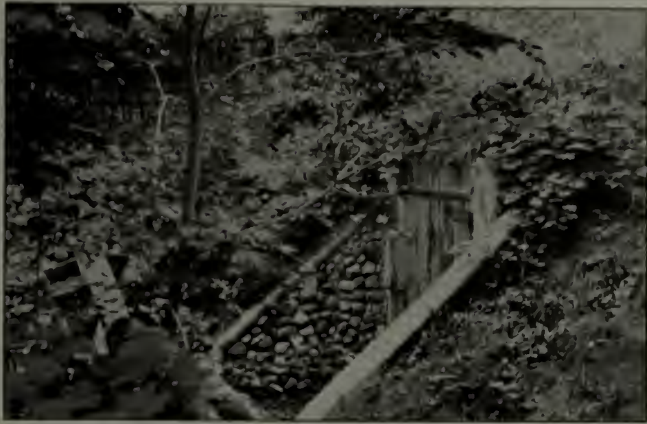
Doorway to a root cellar at Lake Forest, Ill., which has been in successful use for nine years. It is provided with two sets of drain tile, one at the floor line and the other four feet above.
