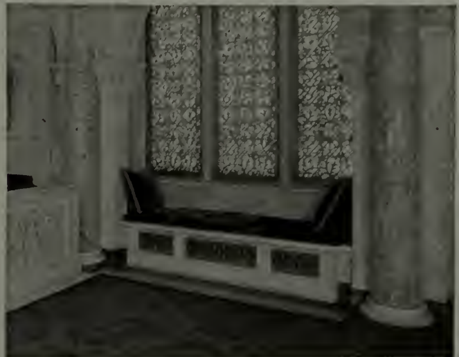
Grille enclosed window radiator in residence of Arthur Curtiss James, New York. Allan & Collens, Architects.
