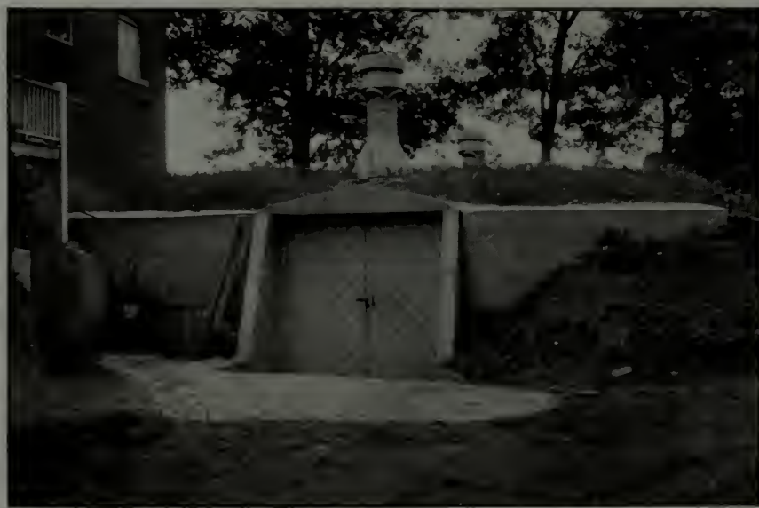
Concrete storage house of Lake Forest University, showing the ventilators above the sodded roof
