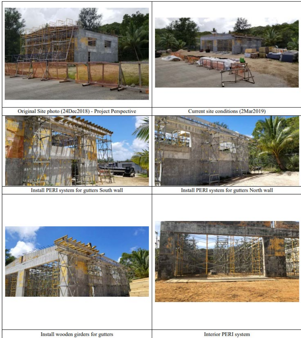
Figure 7 50'x56' concrete storage facility construction (Source: Project Report from the 30 th NCR)
