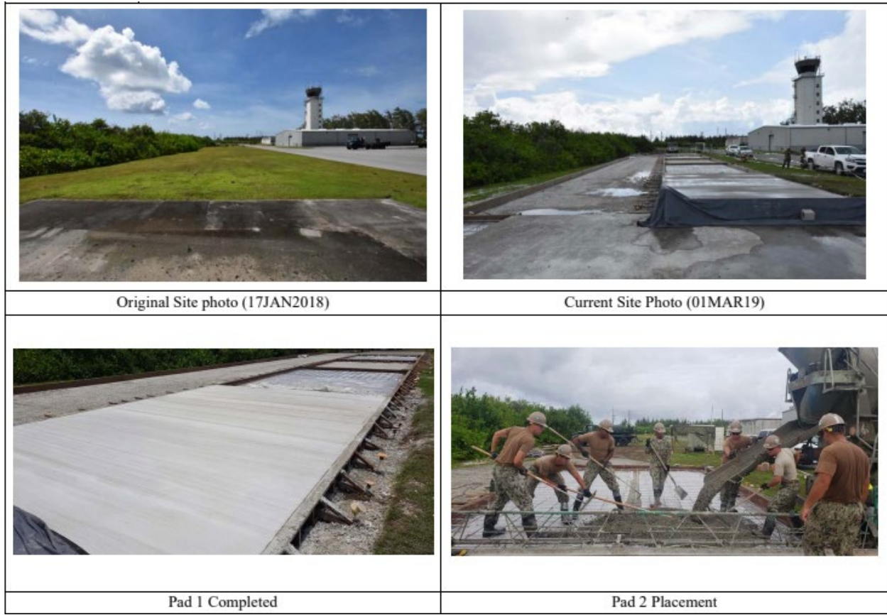
Figure 5 36ft x 205ft x 7in concrete pad construction (Source: Project Report from the 30 th NCR)
