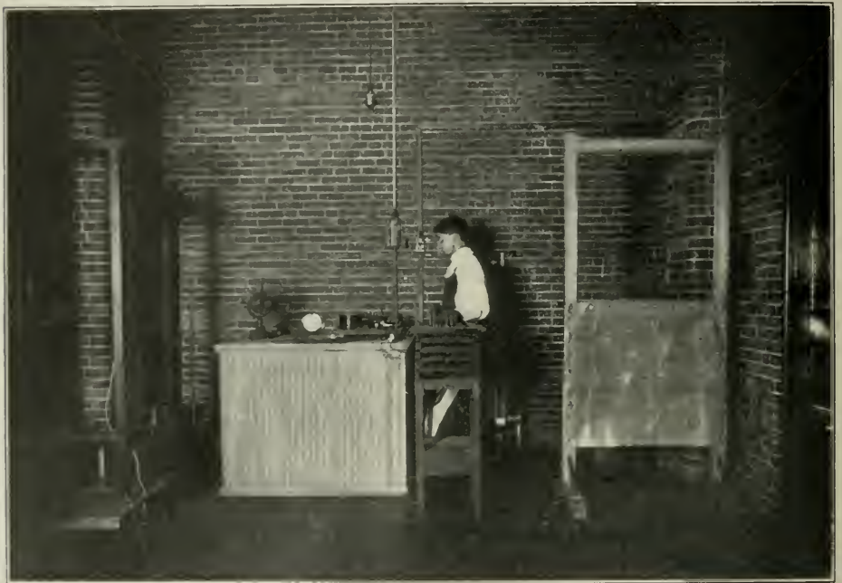
FIG. 181.—X-ray Room of Massachusetts General Hospital, showing closet containing interrupters; on top of closet is the switchboard with knife switches, ammeter, and fuses. Fuses are of lower resistance than main fuses, so that when fuse blows out it may be replaced without the annoyance of going to main board, which may be in the cellar or at some distance. The operator works behind a screen, which, in this picture, has been pushed to one side. (Original.)
