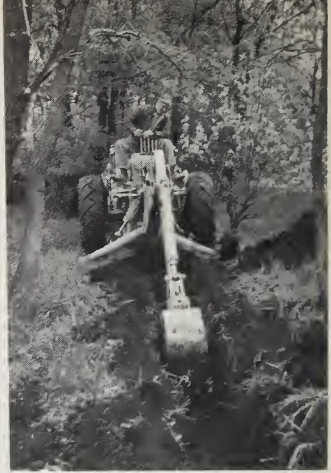
Co-op arranges use of trencher for septic tank hole and disposal field.
