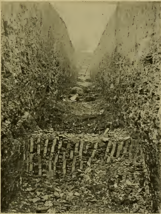
Fig. 3. —Pipe track from Lees Beck to Dalton Gardens Reservoir, showing boulder clay.
