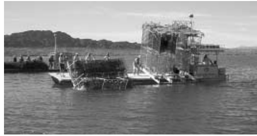
Volunteers installed some 70 acres of fish habitat structures in Lake Havasu in 2002, part of a 10-year effort that resulted in 875 acres of such improvements being added to the lake.
