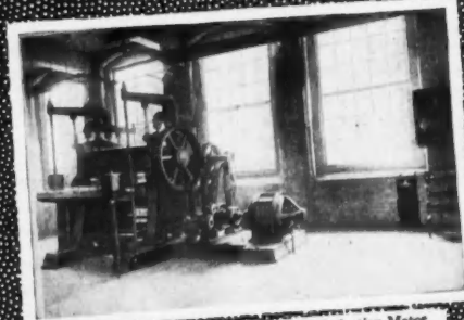
15-h.p., 600-r.p.m., 550-volt Slip Ring Induction Motor and Panel for Plater
