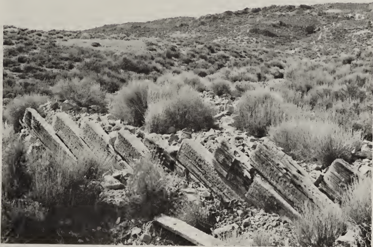
Figure 92: Railroad ties embedded in a wash channel to divert erosion away from the railroad grade. (BLM photo)
