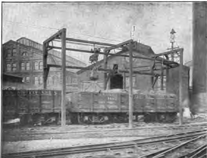
FIG. 2.—STANDARD HOIST, WITH TELPER AND AUTOMATIC DUMPING BUCKET, FILLING CARS. Automatic in operation. Compound curve.
