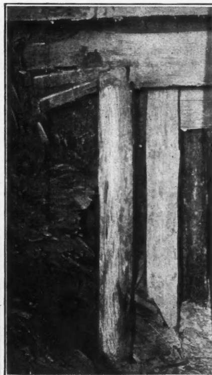
FIG. 5. THE WALLS SOMETIMES SLOUGH AWAY FROM TIMBER
