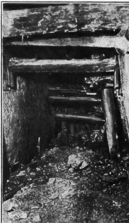
FIG. 4. THE BACK IS CAUGHT UP OVER TOP OF CAVED FILL
