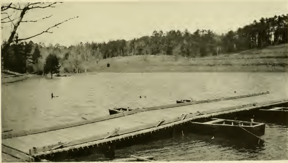
10. SECTION OF PONTOON BRIDGE CONSTRUCTED ON JONES' POND, CAMP SEVIER, GREENVILLE, S. C.
