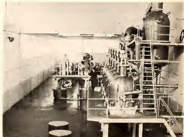
This condenser is part of the new tomato processing equipment now being used in many Portuguese plants.
