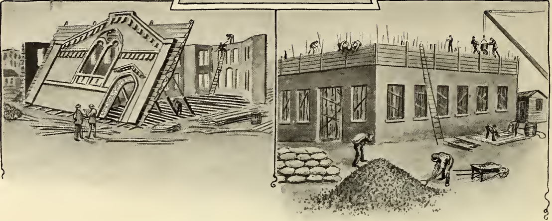
RAISING A CHURCH IN SOLID CEMENT SIDES. (Illustration by courtesy of "Scientific American.")
