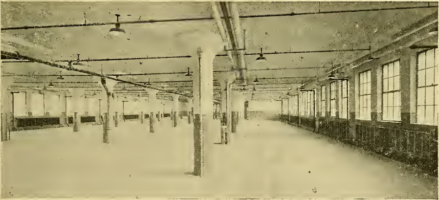
Fig. 6-1. Cast-iron wall radiation on side walls under window, for heating a factory building
