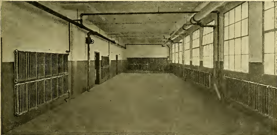
Fig. 10-7. Arrangement of cast-iron wall radiation on side walls of a factory building.
