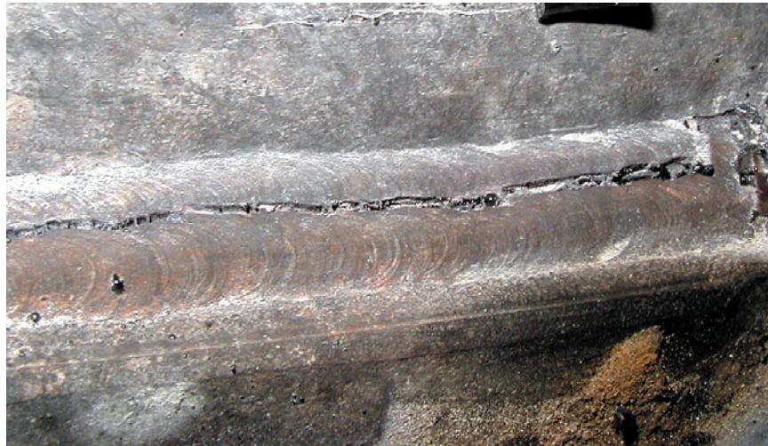
Figure 5. Brittle Fracture of a Ductile Weld Material that Is Constrained – Caused by High Stresses Induced from a Rapid 1000°F Change in Temperature. (Photo Courtesy of Sachs, Salvaterra & Associates, Inc.)
