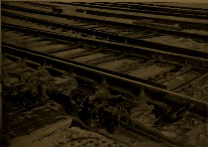
FIG. 416—PNEUMATIC SWITCH MOVEMENT COVER REMOVED.
