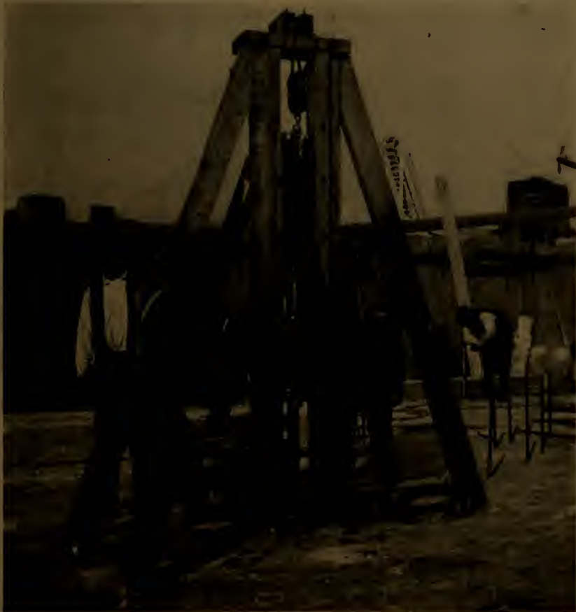
FIG. 377—DRIVING DRIFT PINS BY A COMPRESSED AIR DEVICE. WOOD BORING MACHINE IN THE DISTANCE.
