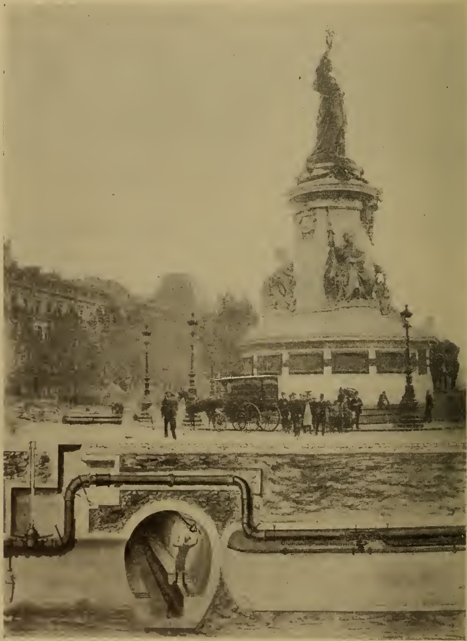
FIG. 64.—PLACE DE LA REPUBLIQUE, PARIS, SHOWING THE COMPRESSED AIR MAIN PIPE LINE.
