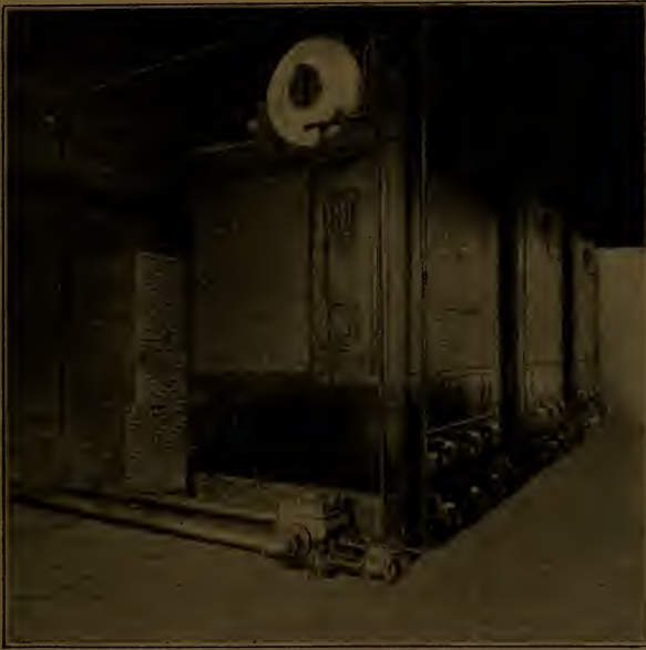
FIG. 319.—THREE HOGAN BOILERS.
