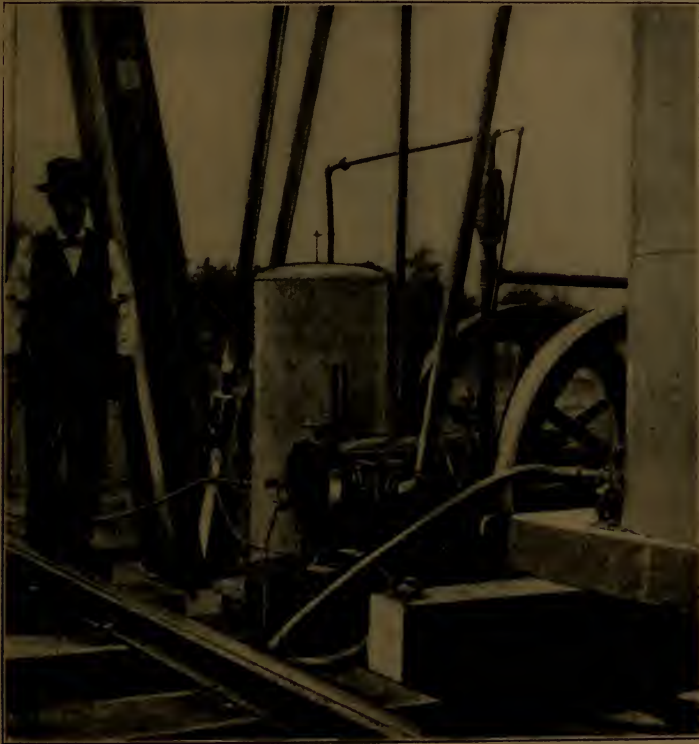
FIG. 51.—GASOLINE ENGINE AIR-COMPRESSING PLANT.
