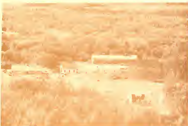
Figure 29. Remaining Fort Egbert buildings, with stabilization work under way on all but the stable, right rear. Open area in center is the old airstrip. (Volz)
