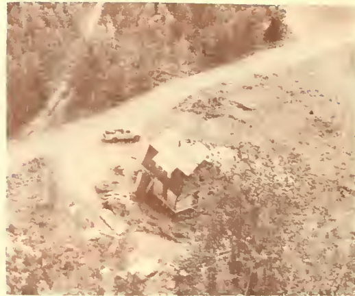
Figure 24. NCO quarters, July 1975, with foundation stabilization completed and building in process of being reroofed. Roofing and replacement of rear shed addition will take place in 1976. (Volz)
