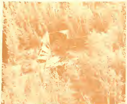
Figure 27. Ruins of second post hospital built in 1906. Remaining walls will be stabilized and potential hazards eliminated. (Volz)
