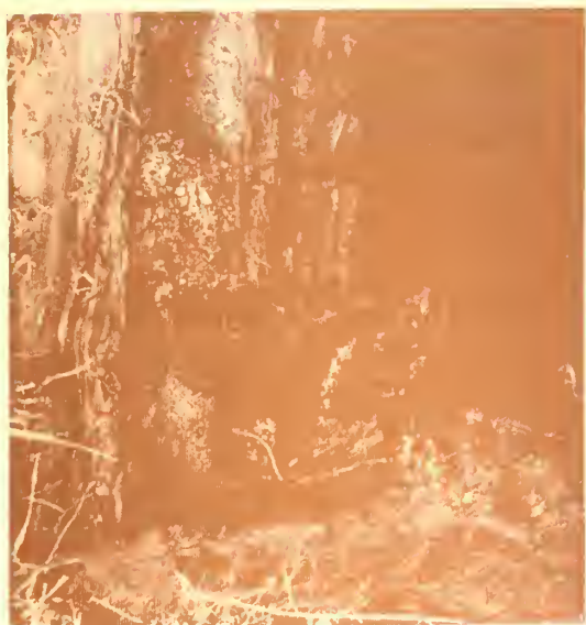
Figure 47. Supporting timbers of the courthouse were totally deteriorated and will require replacement during restoration. (Volz)
