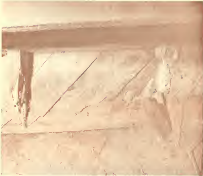
Figure 23. South wall of NCO quarters from cellar. Note absence of foundation, rotted sill studs and line on sheathing indicating an earlier crawl-space soil height. (Clark)
