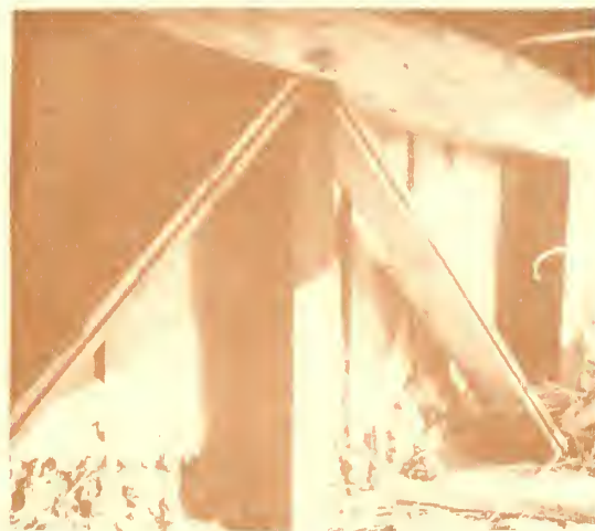
Figure 21. Deteriorated condition of siding on the granary due to direct contact with soil. Note that four to six inches of siding at ground level are totally decayed. (Volz)
