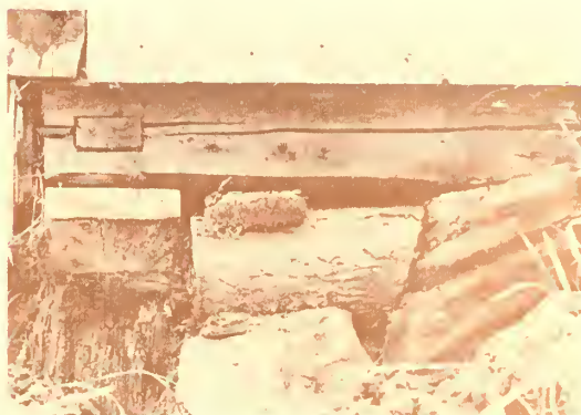
Figure 46. As the courthouse settled and its foundation deteriorated, discarded logs and lumber were used beneath sills and joists to support the structure. (Volz)
