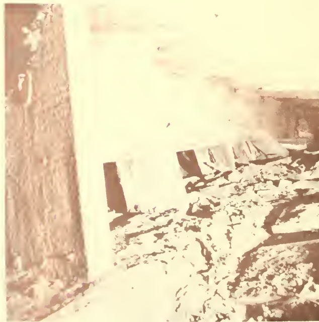
Figure 25. Condition of mule barn foundation at west end. Note angled shearing of post top in foreground. (Clark)
