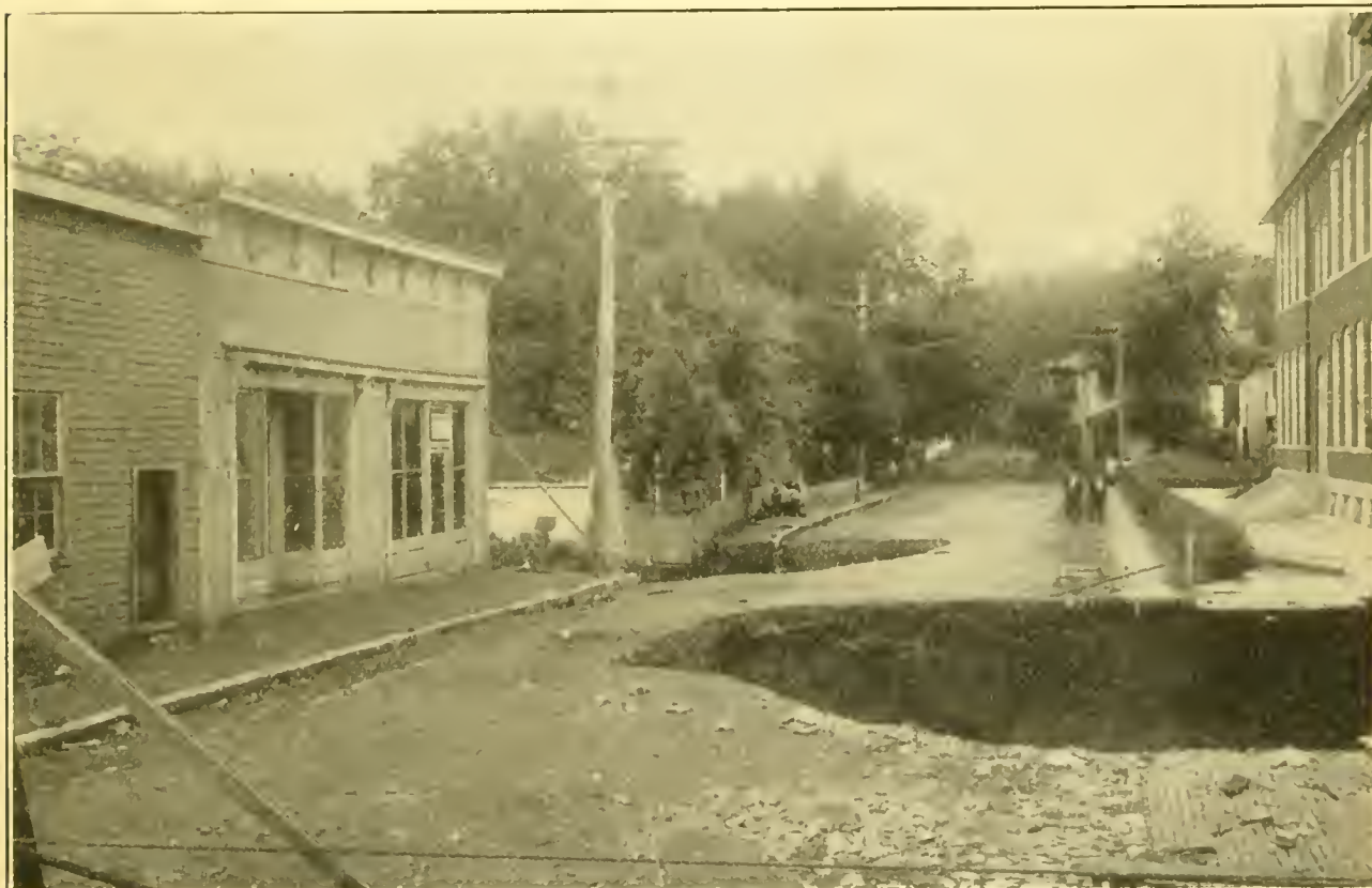
Fig. 2 View of two of the holes in Baldwin Street, taken after the disappearance of the house shown in Fig. 1.
