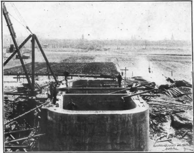
FIG. 9. TOP OF COMPLETED SHAFT, SHOWING FARM LANDS, SUSQUEHANNA RIVER, AND WILKES-BARRE, PENN., IN BACKGROUND
