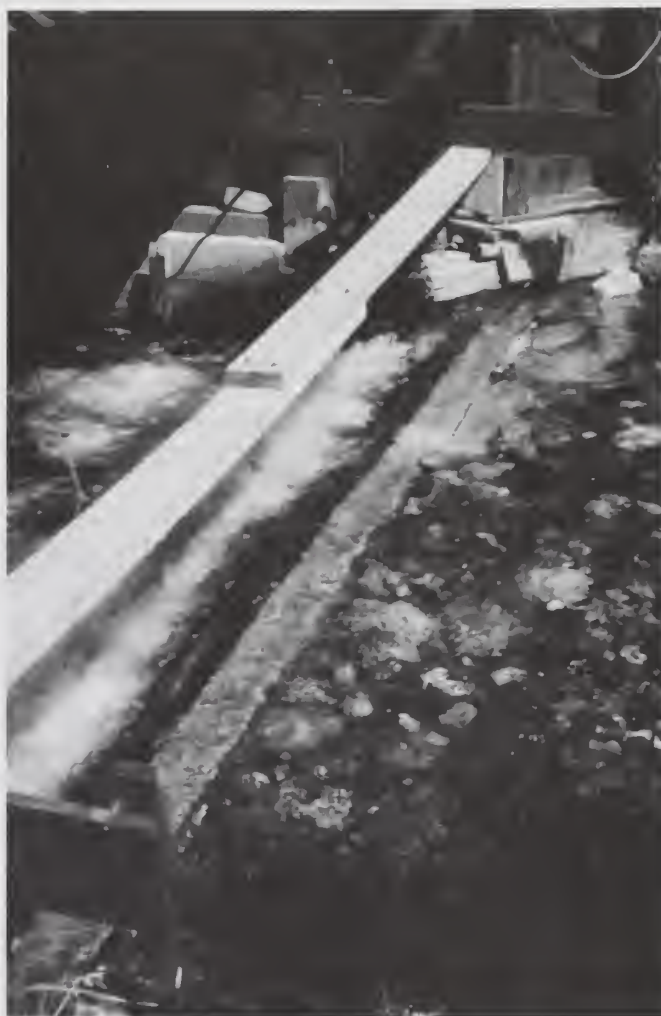
Figure 4.3 – Detector log is installed flush with the river bed and spans the entire stream width.
