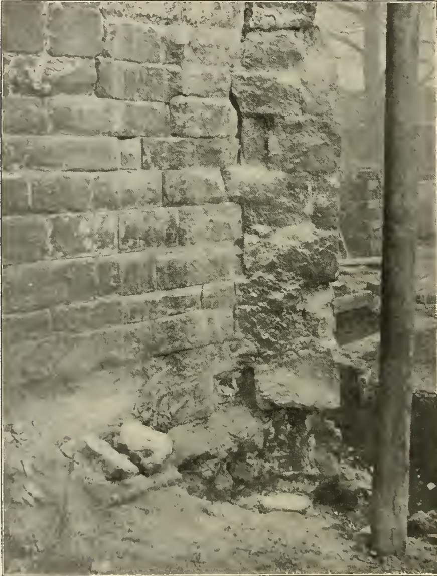
The South-East Buttress of the Chancel showing the fracture and settlement.
