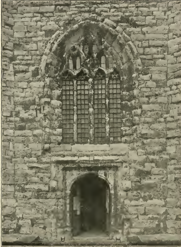
Detail of the West Doorway and Window, before the restoration, showing the decayed condition of the work.
