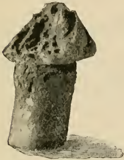
A CORRODED RIVET.
