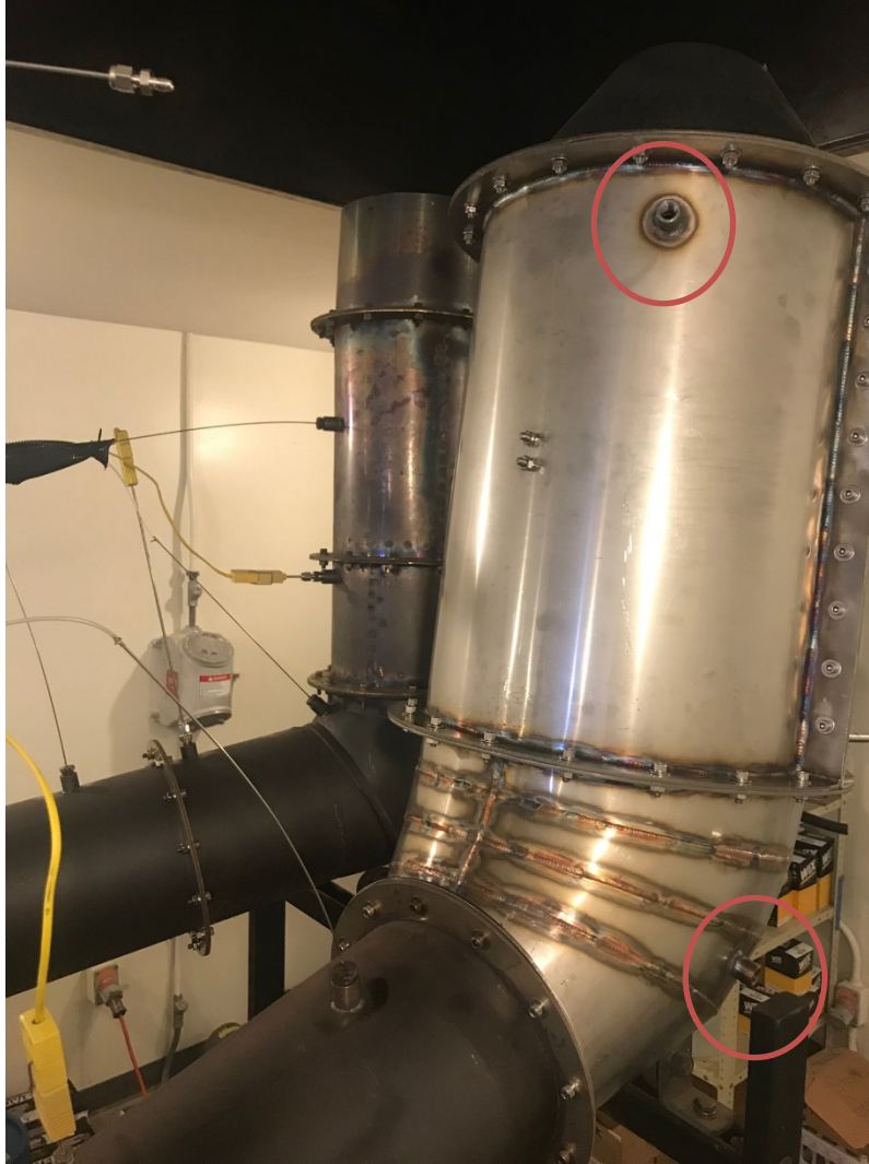
Figure 23. Installed Heat Exchanger 2
