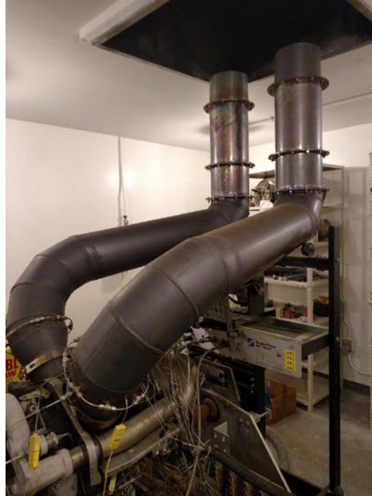
Figure 4. NPS Gas Turbine Test Cell Exhaust Duct Setup. Source: [6].
