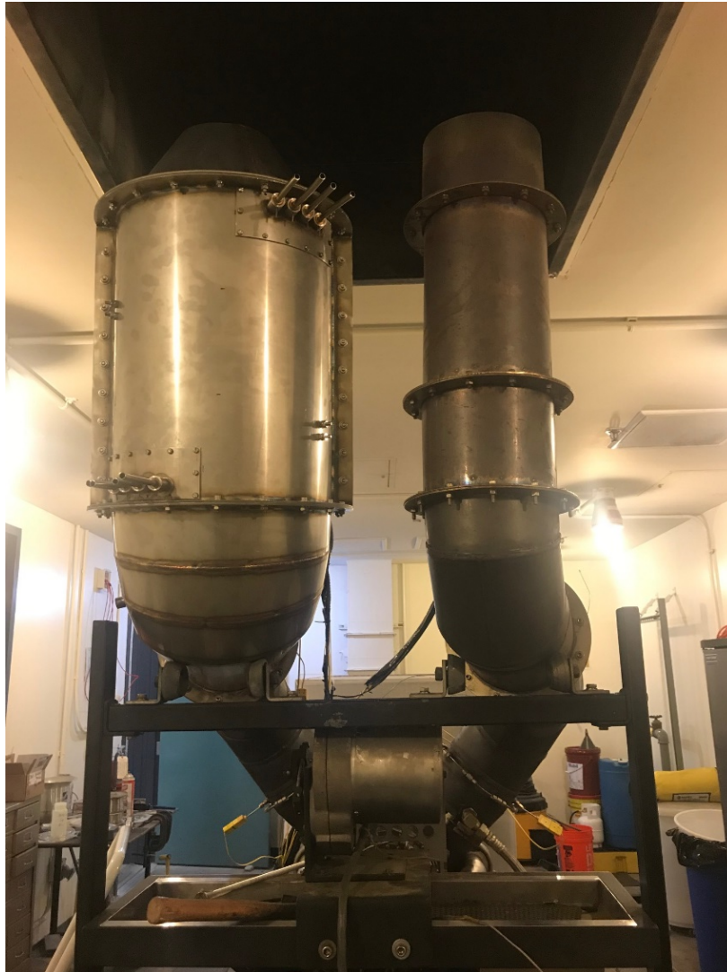
Figure 22. Installed Heat Exchanger 1
