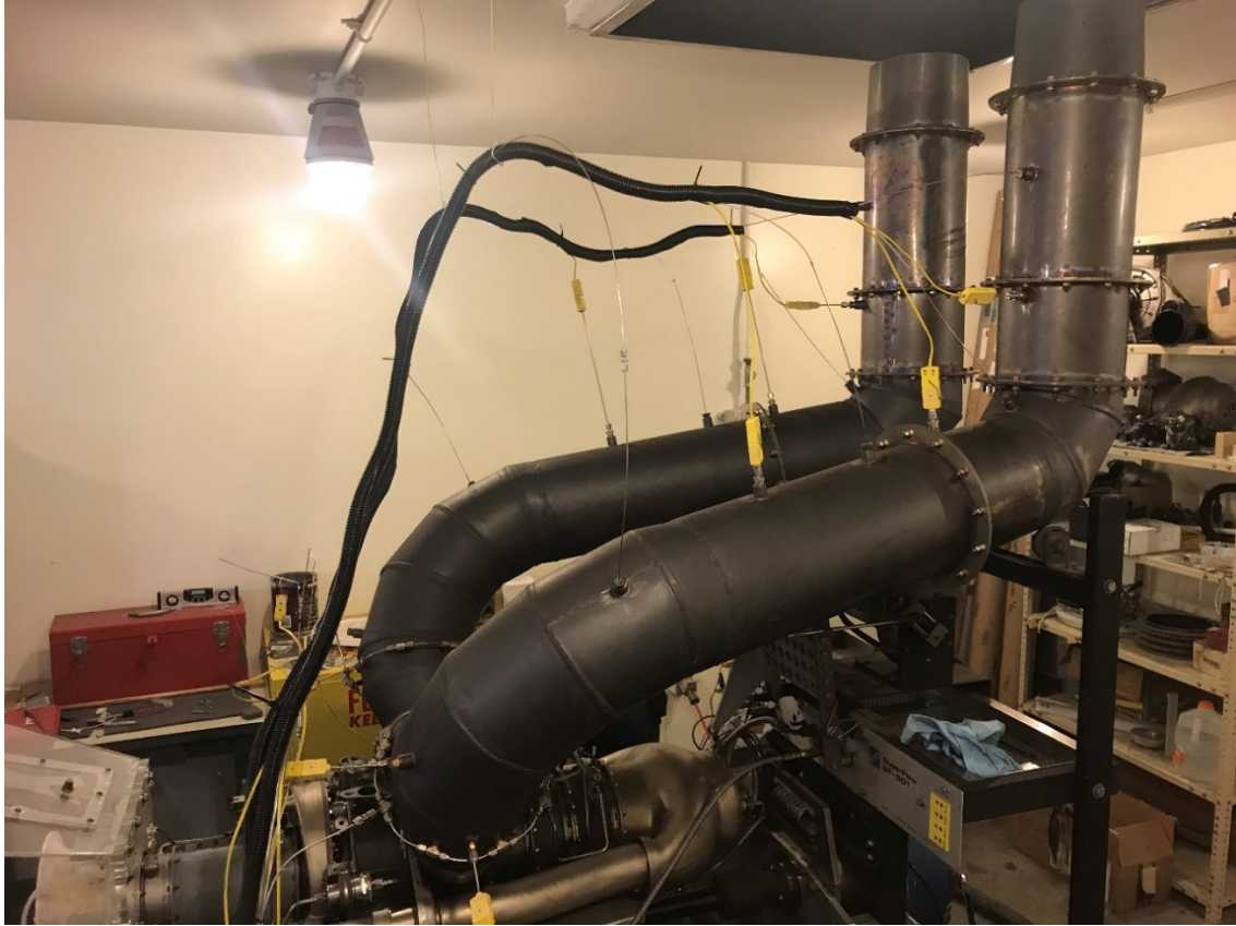
Figure 9. Locations of Pressure and Temperature Probes Along Stacks
