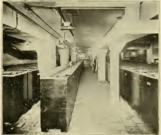
REAR PORTION OF BATTERY ROOM.
