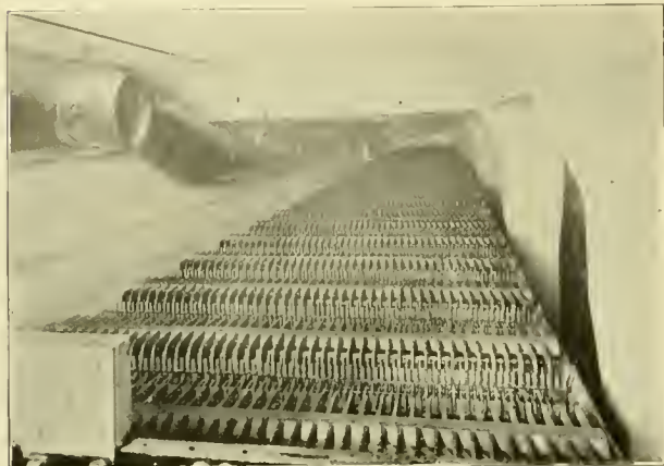
VENTILATING DUCTS IN BATTERY ROOM.
