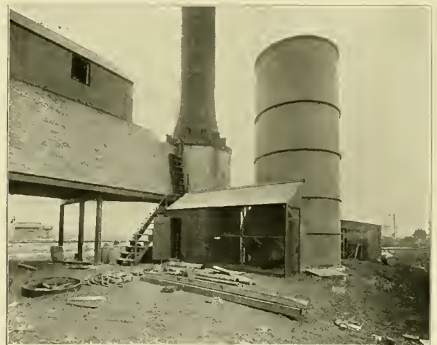
FIG. 3.—COOLING TOWER AND ECONOMIZER.
