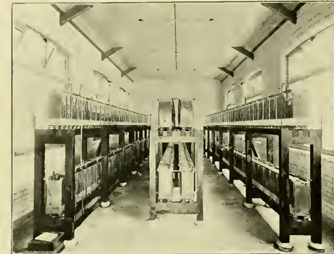
STORAGE BATTERY ROOM.
