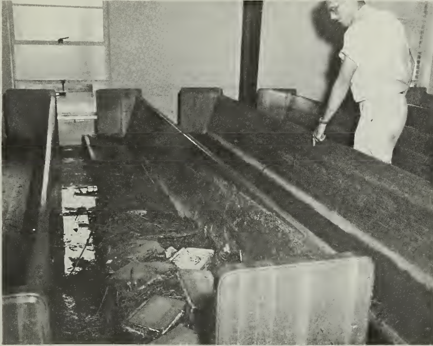
Newly furnished and redecorated church received extensive flood damage. Note water-soaked song books and debris in pews. The raging floodwater almost overtopped the pews. Another church was completely destroyed.
