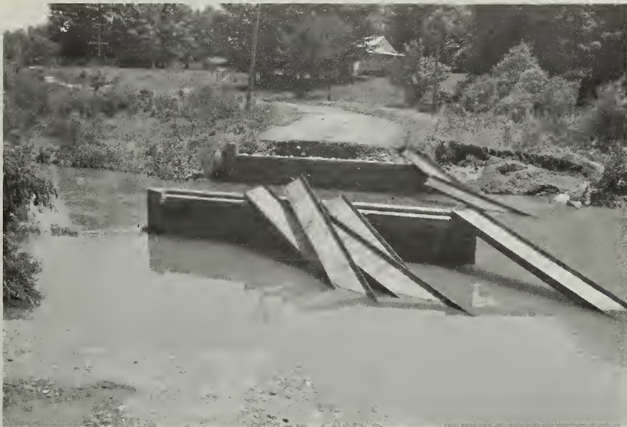
This is typical flood damage to city and county roads and bridges.
