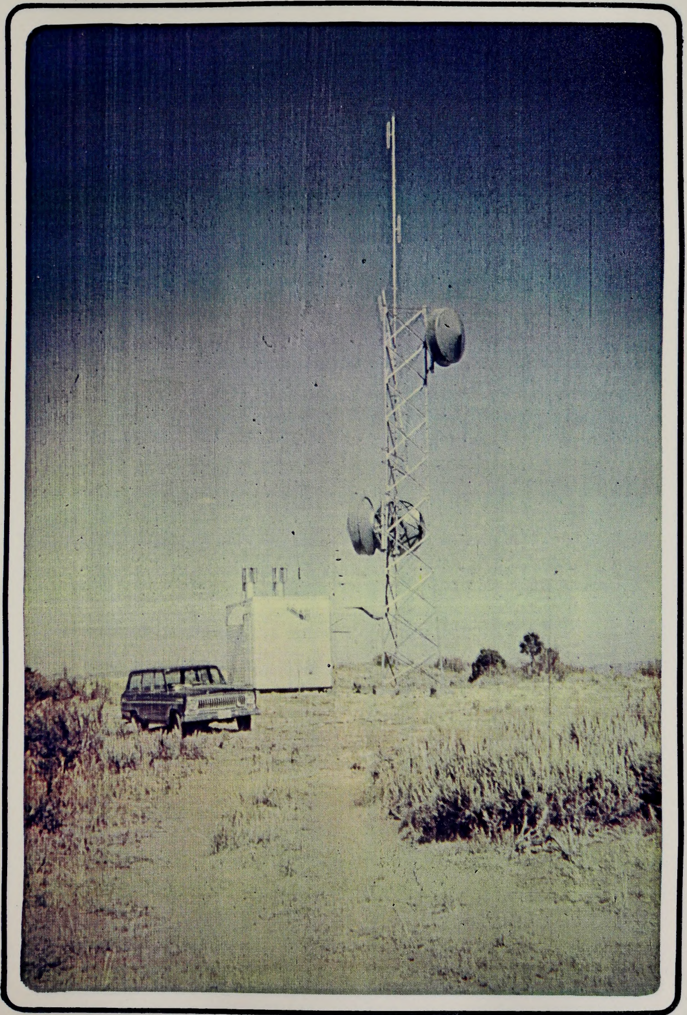
Figure C-9 - The microwave station of the Western Slope Gas Company on Kendall Peak.
