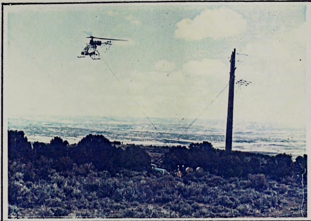
Helicopter has just left ground with conductor wire to start the stringing operation. Note conductor spool with braking winch on ground.
