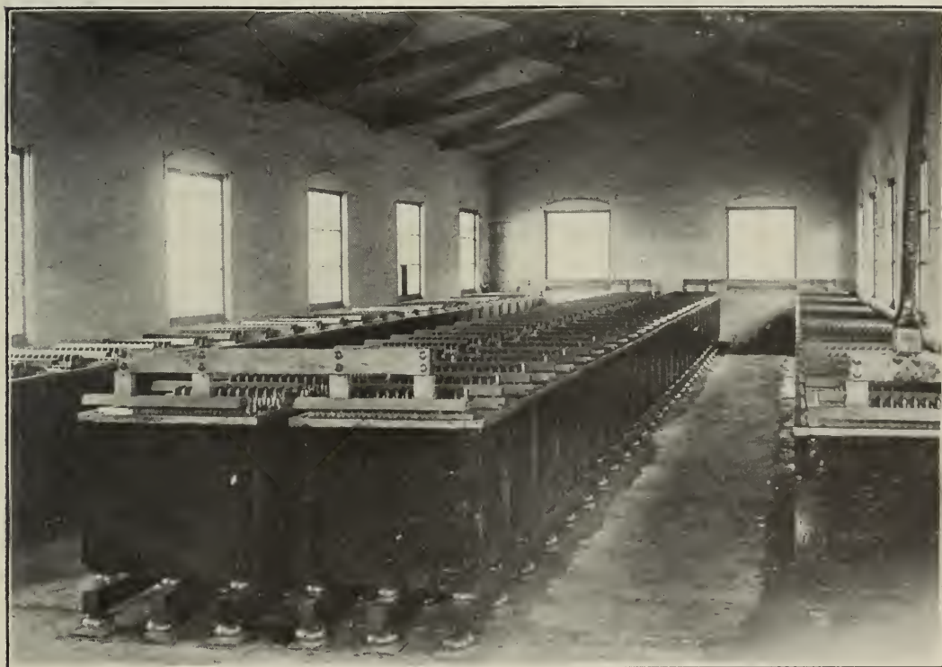
FIG. 13. BATTERY ROOM, ROLLING MILL PLANT, CAMBRIA STEEL CO. Floating battery, Bijur "high-duty" type. Regulating capacity, 600 k. w. General Storage Battery Co.
