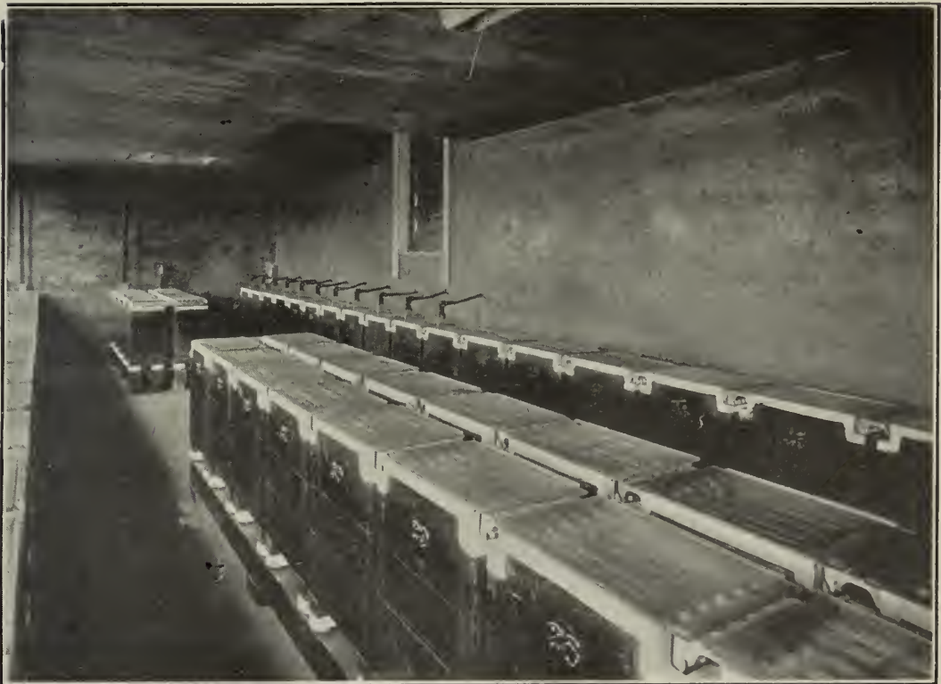
FIG. II. BATTERY INSTALLATION, GOULD STORAGE BATTERY CO.
