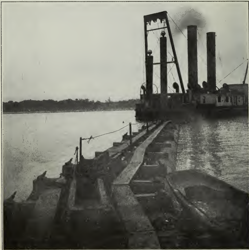
PIPE LINE OF 30-INCH HYDRAULIC DREDGE BUILT FOR THE COMMISSIONERS OF LINCOLN PARK, CHICAGO.
