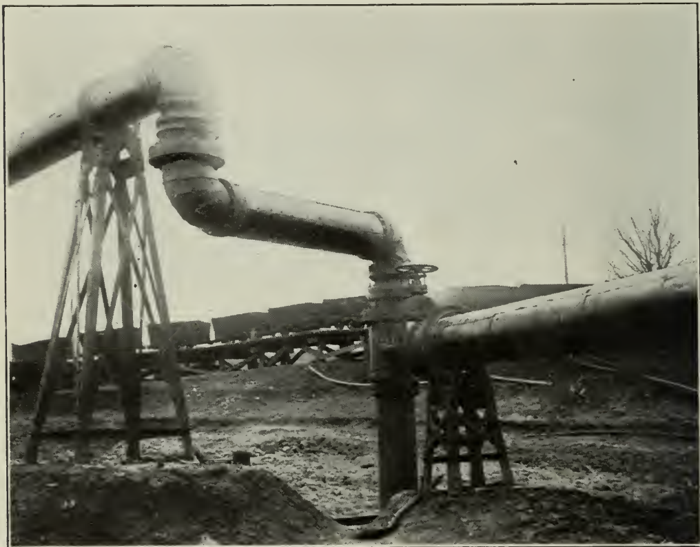
SWIVEL EXPANSION JOINTS AT MIDDLE OF THE LINE.
